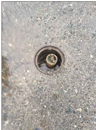
4. Offsite well MW-5 damaged; installed new well cap.
