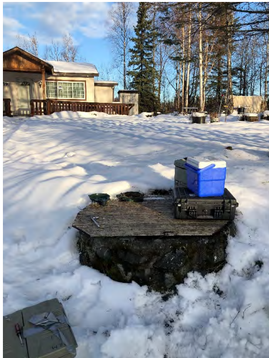
Photo 2: Drinking water well located at 22179 Birchwood Loop Road, Chugiak, Alaska. Covered with an unsecured plywood board; facing southwest. 11/15/2018 11:42.
