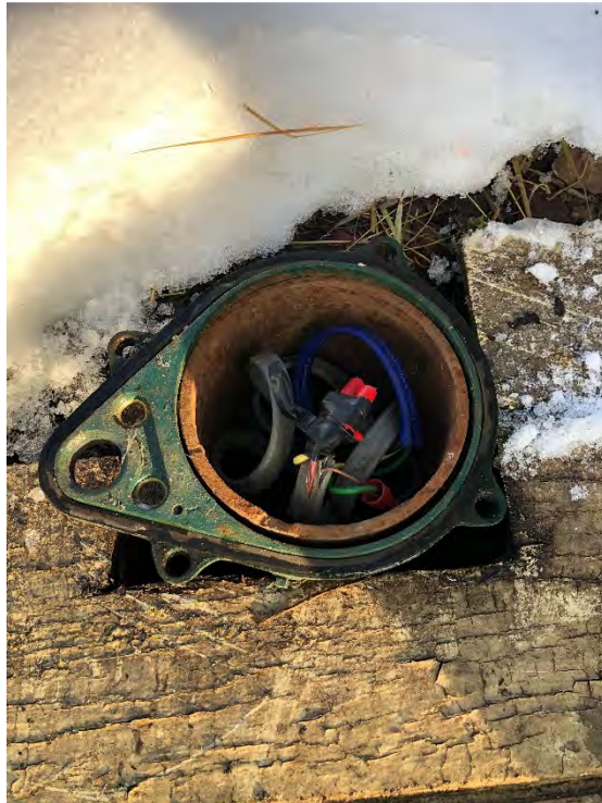
Photo 1: Drinking water well located at 22179 Birchwood Loop Road, Chugiak, Alaska. 11/15/2018 11:42.
