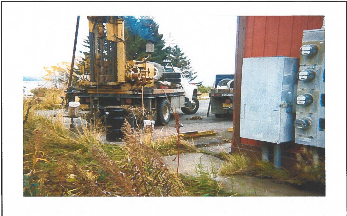
Photo 1: A view of the drill rig during Monitoring Well B12MW installation; looking southwest (October 2003).
