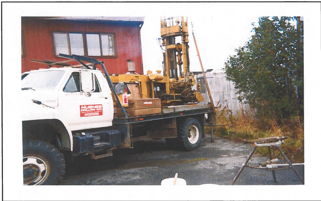
Photo 2: A view of the drill rig during Monitoring Well B12MW installation; looking northeast (October 2003).
