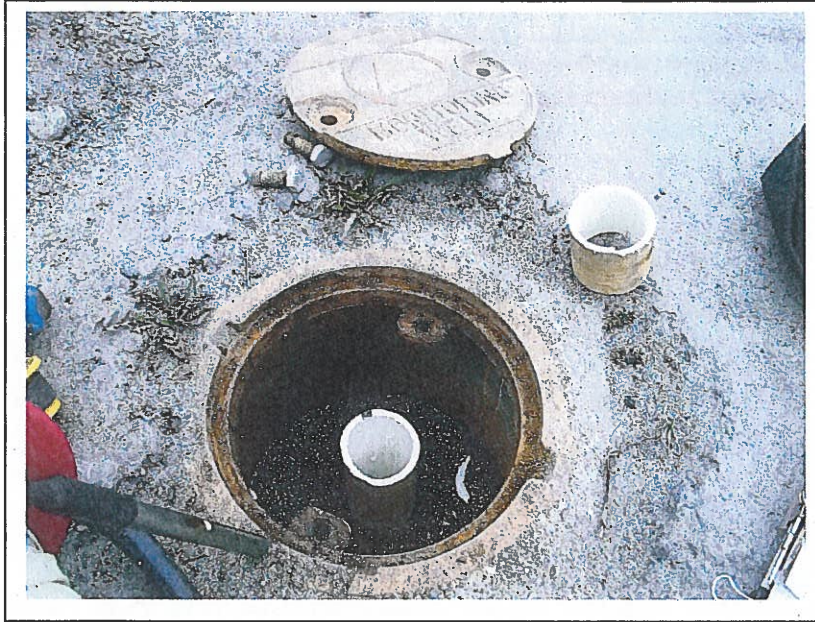
Photo 1: A view of Monitoring Well MW-4 after the well casing was cut down to allow clearance for the well plug (May 21, 2013).
