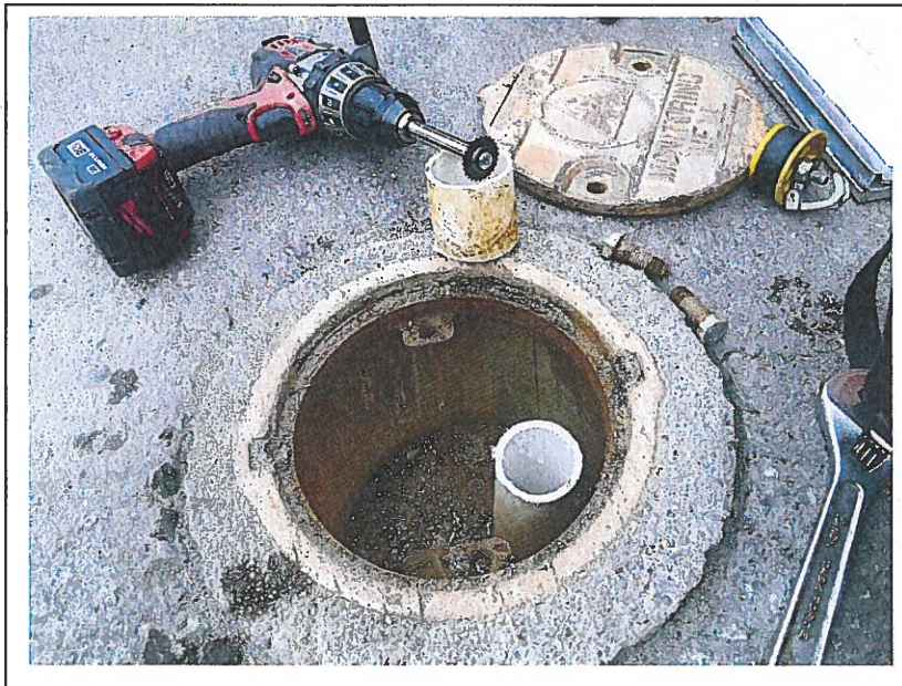
Photo 2: A view of Monitoring Well MW-7 after the well casing was cut down to allow clearance for the well plug (May 21, 2013).
