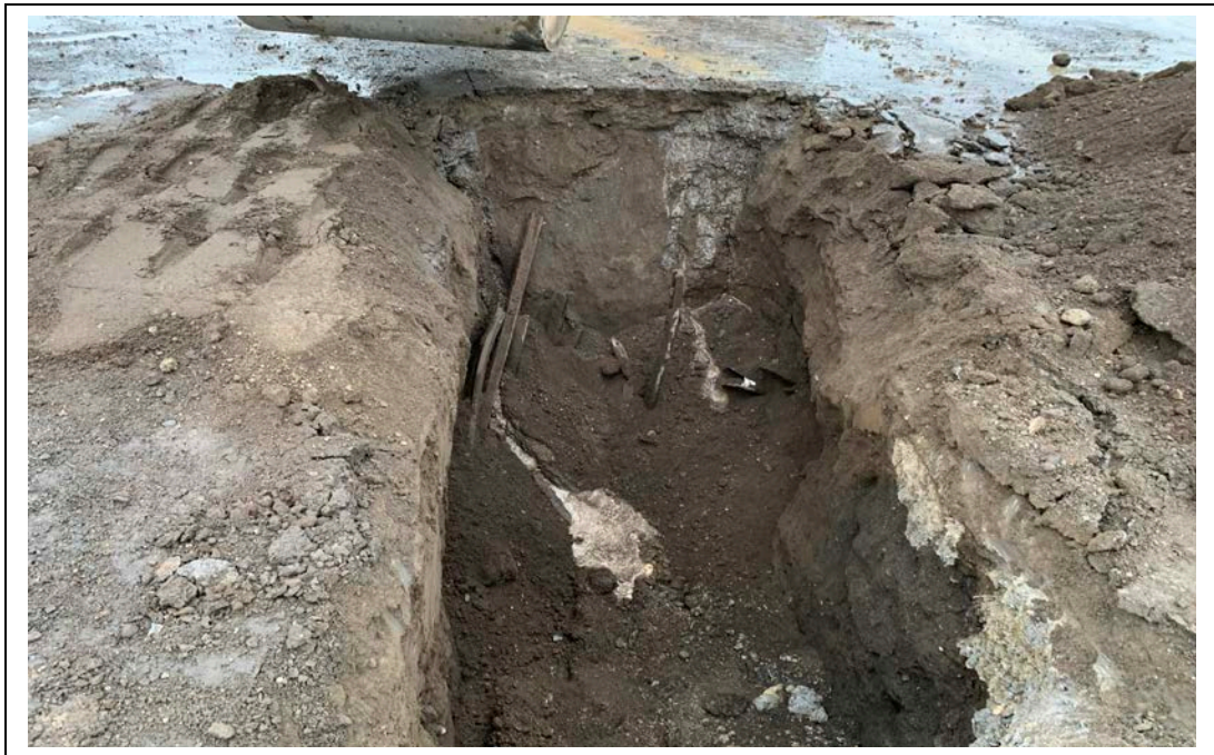
Photo 2: Looking south into Test Pit TP1. Metal debris were encountered between approximately 4 to 6 feet bgs. (November 5, 2020)
