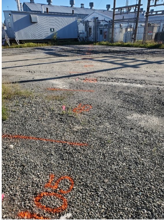
Photo 1: Boiler Building Trench Excavation –Trench transect divided into 10-foot sections, facing HOA Building.
