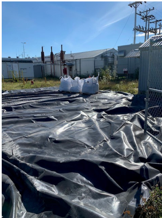
Photo 4: Boiler Building Trench Excavation – Supersacks placed on the liner inside the perimeter fence.
