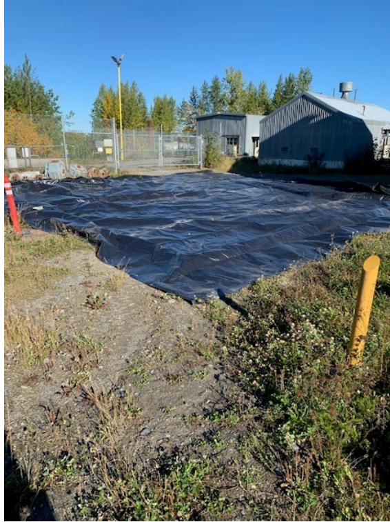
Photo 3: Boiler Building Trench Excavation – Liner inside the perimeter fence for supersack storage.
