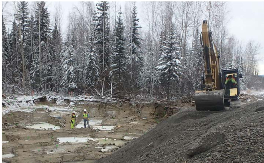
1,350 gallons of jet fuel from a truck rollover accident were excavated in Fort Wainwright, Alaska.
