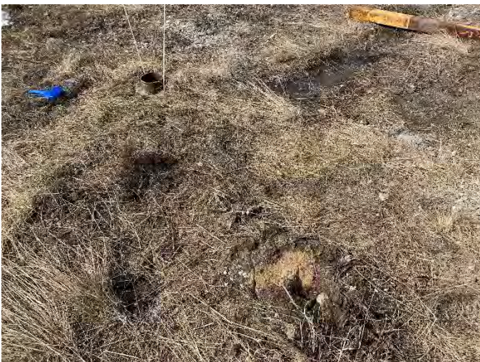
Photo 3: Decommissioning activities complete at MW-8 in accordance with Section 6.2 of the Work Plan. Sand and bentonite filling remaining borehole in foreground.
