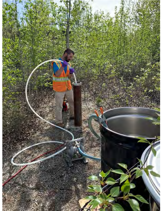
Photo 4: Redeveloping MW-32 using an air diaphragm pump and surge block prior to sampling.
