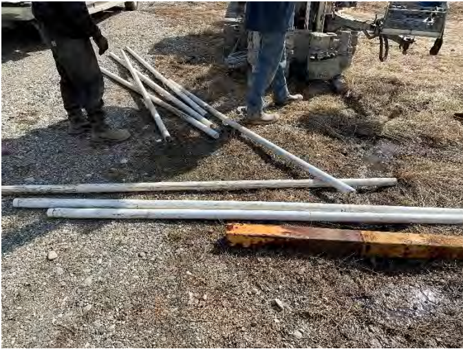
Photo 2: Decommissioning MW-8: constructed of 2-inch PVC casing to a depth of 80 feet, with a 5-foot steel stick-up monument.
