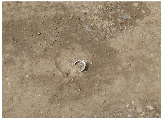
MW-12 before repair.
