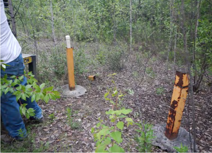
MW-5 (left) and MW-4 (right) before repair.
