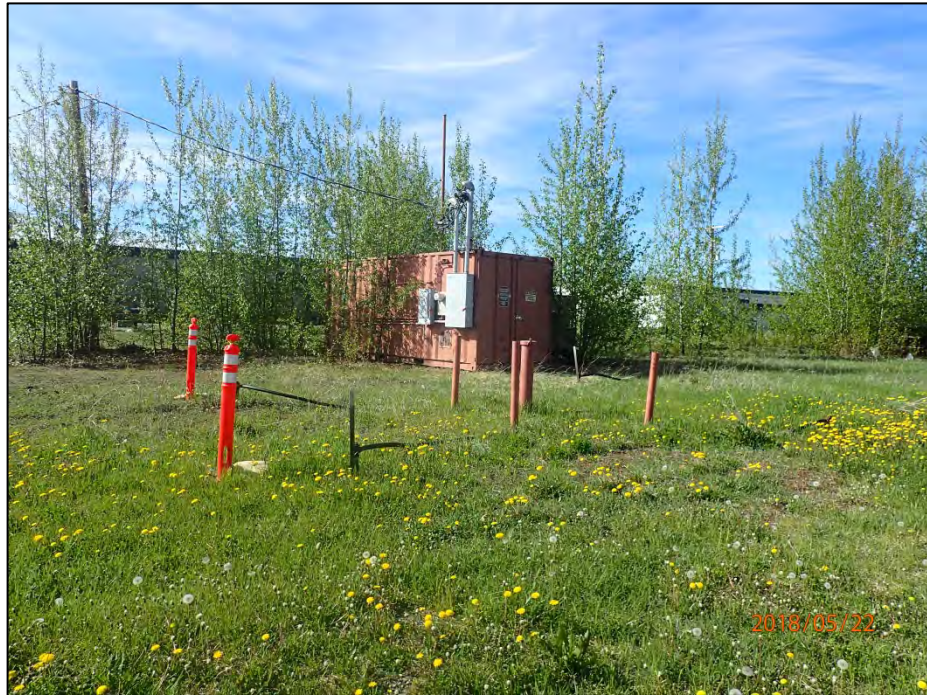
Monitoring well AP-9684 and treatment system connex (View to South).
