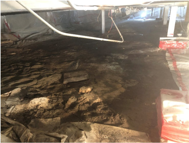
Photo 1. Portion of Bamboo Panda crawlspace where the vapor barrier was removed and replaced. Facing northwest.
