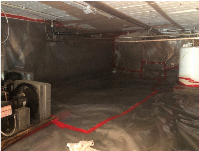
Photo 2. Bamboo Panda crawlspace vapor barrier repair near the refrigeration unit (on left). Looking southwest.
