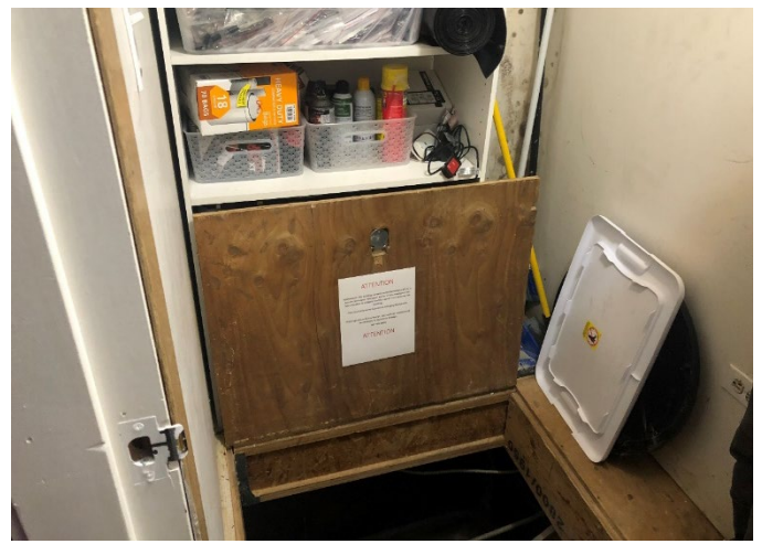
Photo 5. Sign regarding vapor barrier posted on crawlspace access hatch.
