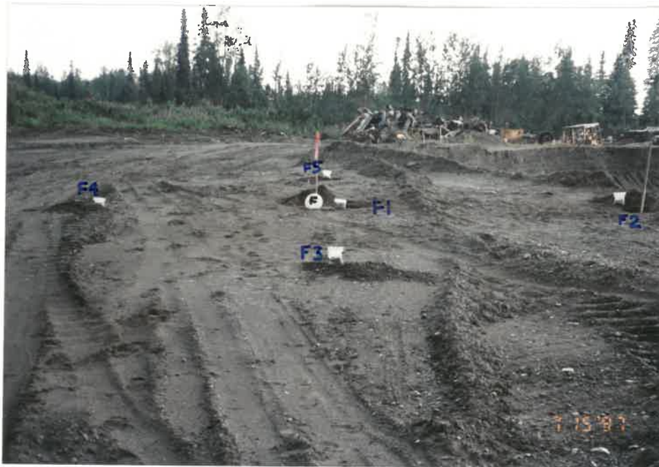
Looking west at area F - test holes F1, F2, F3, F4 and F5 note: Active pit area is in the upper right quadrant
