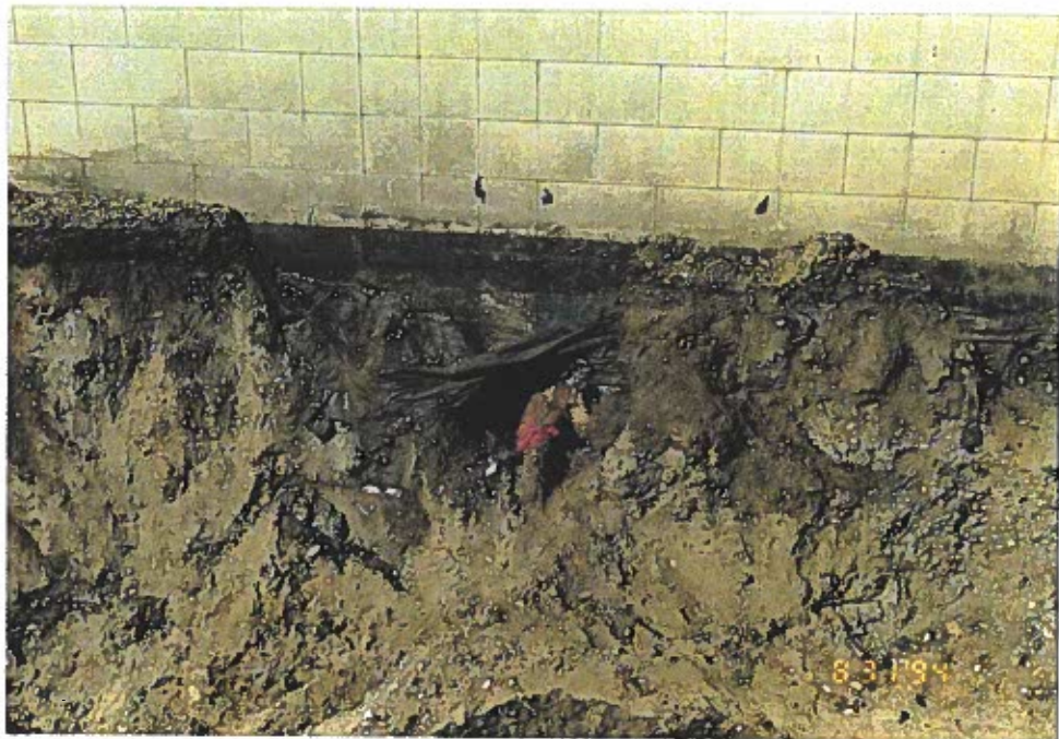
Photo 2: View of sub-floor drain piping exiting the garage building at the excavation edge.
