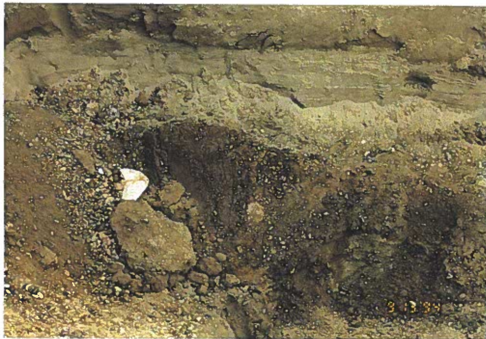
Photo 6: View of excavation bottom directly beneath the former location of the gasoline tank.
