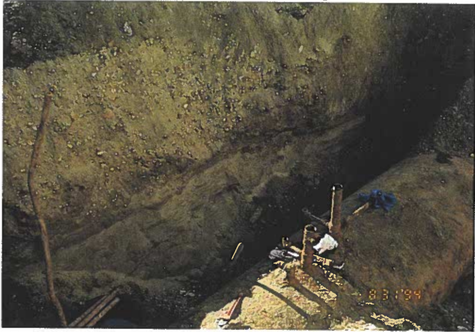
Photo 1: View of the two 500-gallon used oil tanks in place. Piping has been removed.
