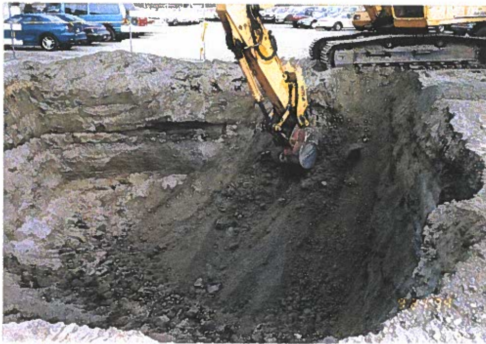
Photo 13: View of soil removal from the southeastern corner of the excavation during contaminant tracking.
