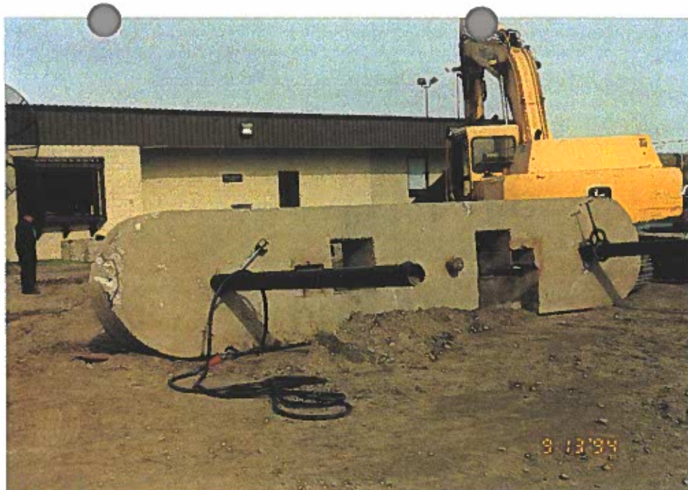
Photo 1: A concrete dispenser island, formerly located directly over the end-to-end tanks, was removed during initial site work.
