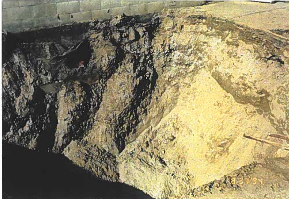
Photo 8: View showing general soil types encountered during excavation activities in used oil tank area.
