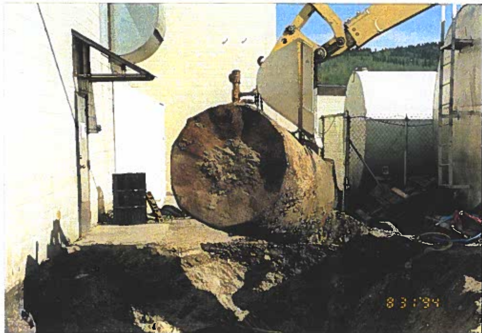
Photo 6: View of UST No. 2 during removal. Note concave shape of tank end.
