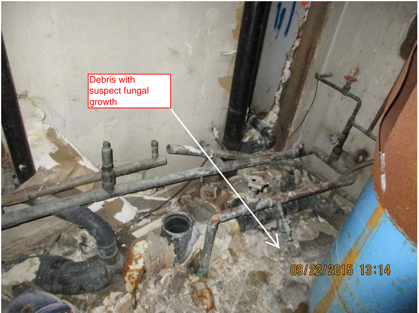
Figure 8 – Suspect fungal growth on gypsum wall board debris on the floor of the mechanical room.
