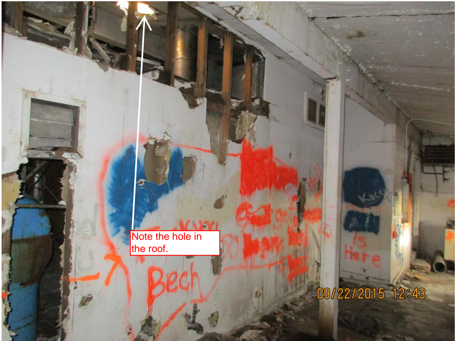
Figure 2 – The wall separating the laundry room and mechanical room. Note the hole in the roof above the mechanical room.
