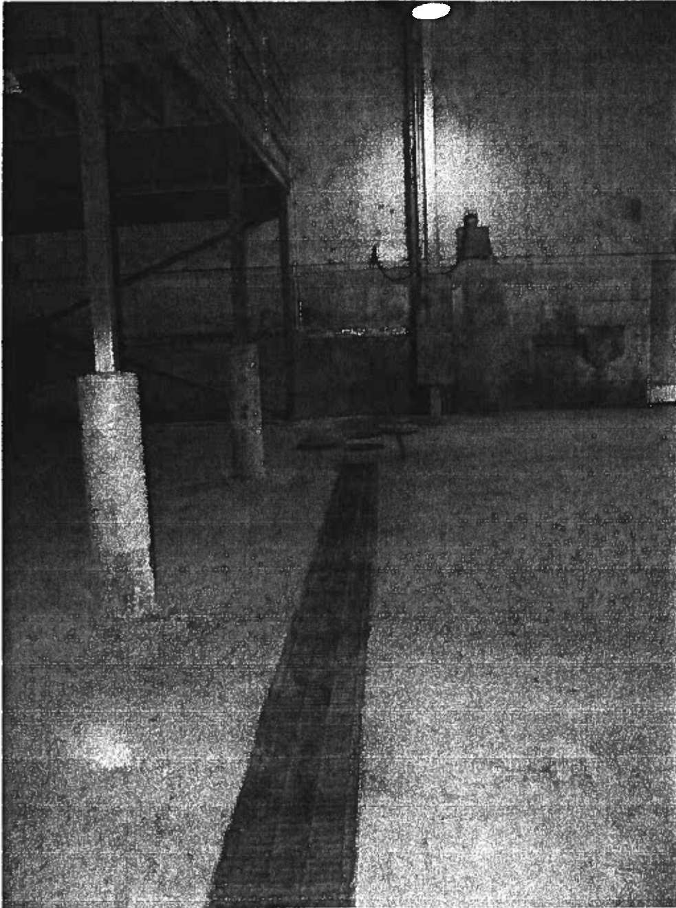
PHOTO 2: Strip floor drain and oil/water separator/sediment trap (covers removed) in South bay of warehouse/shop building.
