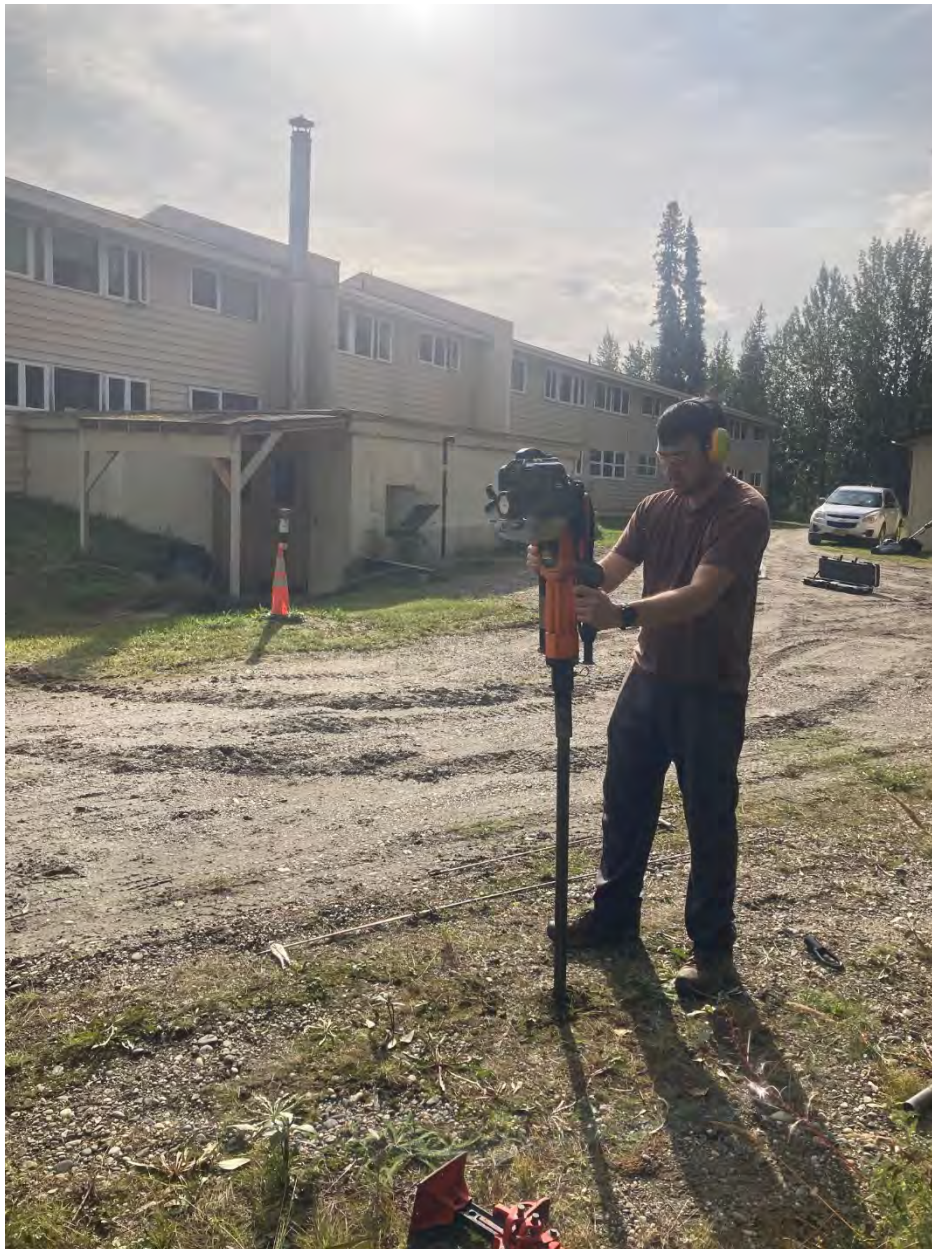
Photo 4. Downgradient borehole location, with Geoprobe LB sampler rod being driven with Skidril G20D powered driver by ADS principal chemist Rodney Guritz
