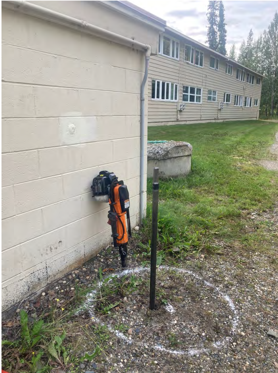
Photo 3. Release location marked near boiler room, with Geoprobe LB sampler rod driven with Skidril G20D powered driver
