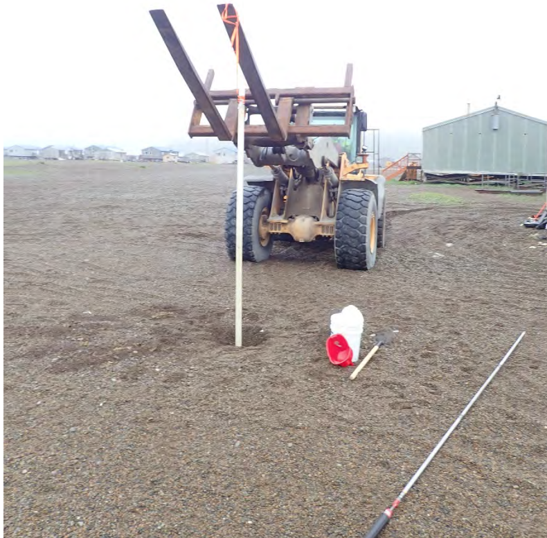
Photograph 2: Well 16GAMMW02 being removed by SM using loader. Well screen has been knocked from bottom of well using slide hammer attachment in bottom right of photo. Well PVC has been filled with bentonite pellets before removing to act as a tremie pipe.
