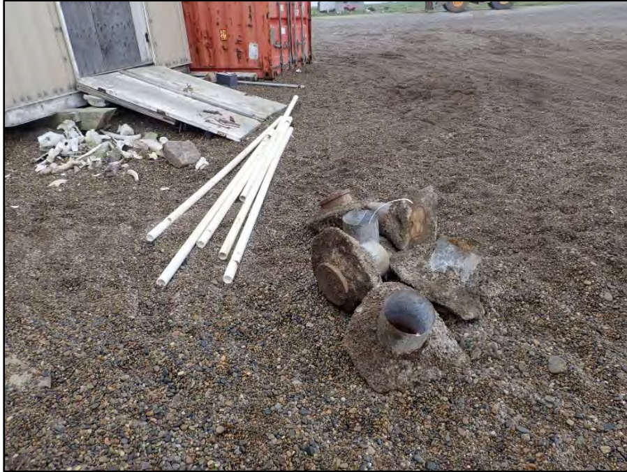
Photograph 3: Six flush mount wells (16GAMMW01, -02, 1-03, -04, -06, -07), casings, and lids removed and ready for disposal.
