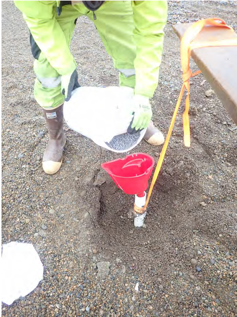
Photograph 1: Well 16GAMMW02 with concrete casing and lid removed. Well PVC strapped to loaded fork blade. JP pouring bentonite pellets into well before removal.
