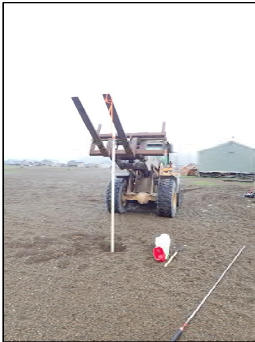
Photograph 2: Well 16GAMMW02 being removed by SM using loader. Well screen has been knocked from bottom of well using slide hammer attachment in bottom right of photo. Well PVC has been filled with bentonite pellets before removing to act as a tremie pipe.
