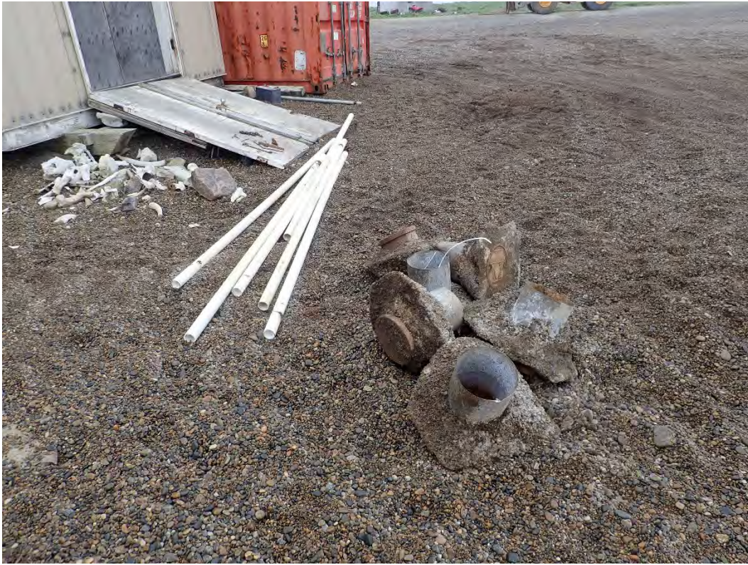
Photograph 3: Six flush mount wells, casings, and lids removed and ready for disposal.
