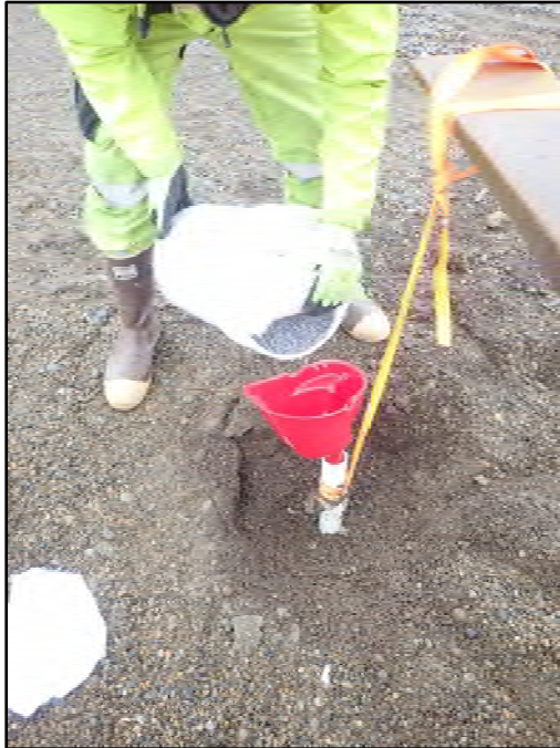
Photograph 1: Well 16GAMMW02 with concrete casing and lid removed. Well PVC strapped to loaded fork blade. JP pouring bentonite pellets into well before removal.
