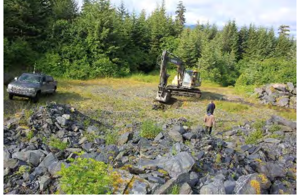
Photo showing TH27 at the Mile 6.5 Rock debris Area.
