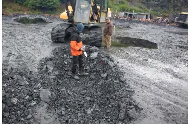
Photo showing TH21 dug in center of road at the Sort Yard Circle.
