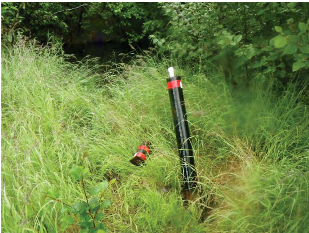
Photo 6: Site OT001, Subarea PT1, well PT1SB04; view of pre-repair condition.
