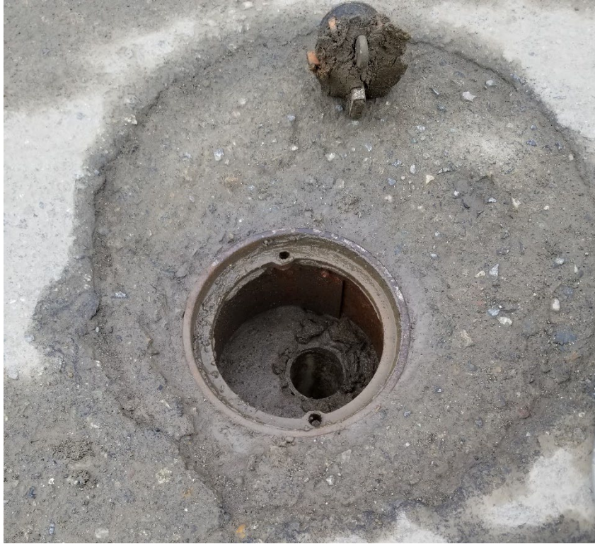
Photo 3: Silt accumulated in the surface monument of MW5. September 10, 2021.
