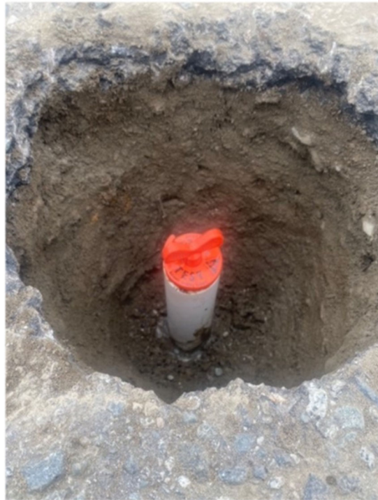
Photo 4. MW-5. Polyvinyl chloride (PVC) was cut down to accommodate frost jacking.
