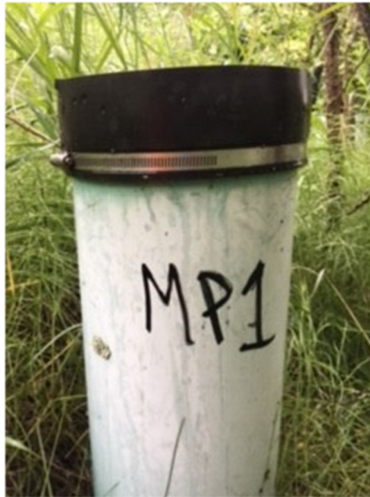
Photo 2. Monitoring Point (MP)1. MP2 through MP4 are of similar construction. MP1 and MP4 had a petroleum sheen on the groundwater and a petroleum odor was observed. MP2 was dry but a petroleum odor was observed.
