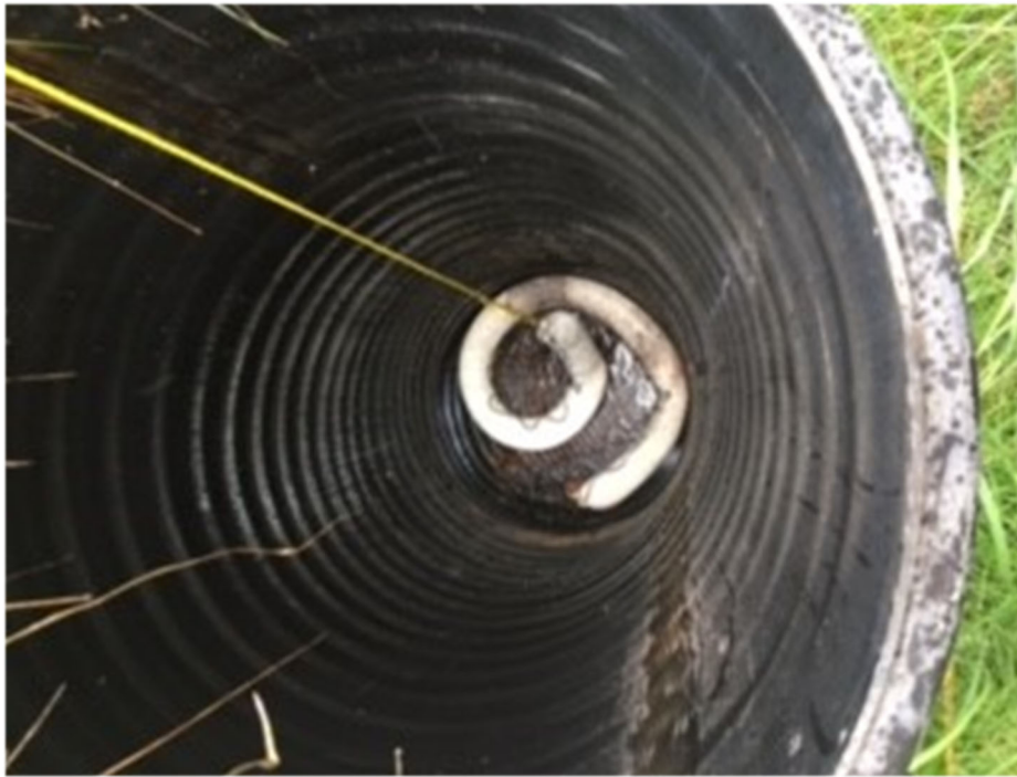
Photo 1. Sump 1 located at the northern end of the recovery trench. Sump 2 is of similar construction and is located at the southern end of the recovery trench. In both sumps a petroleum sheen was present on the groundwater and a petroleum odor was observed.
