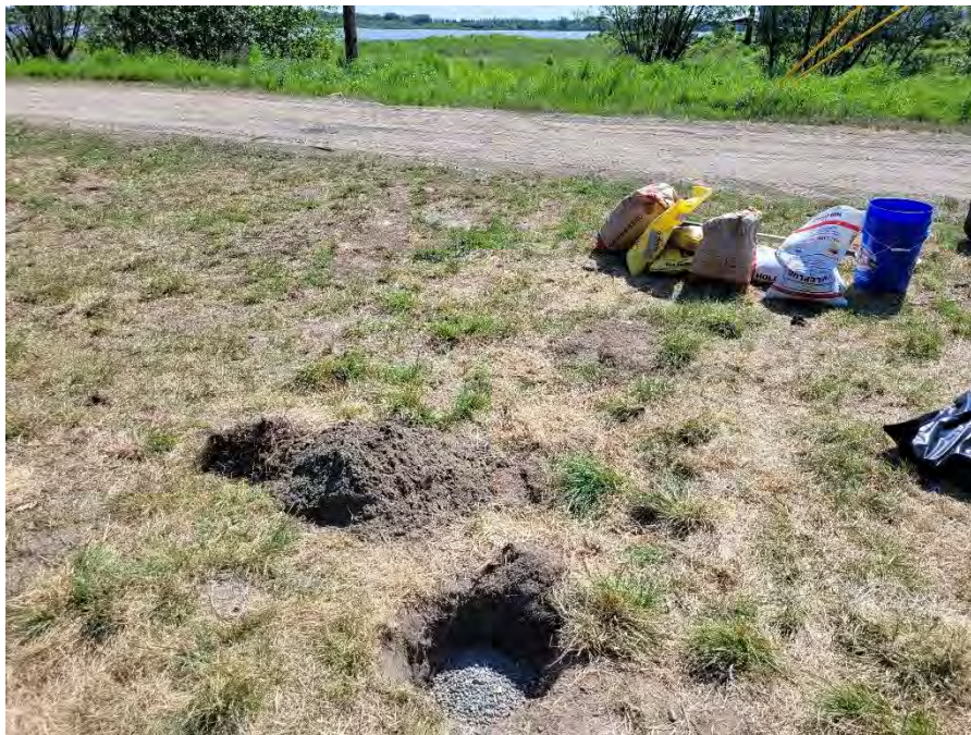
Photograph #2 – 6 June 2022. The decommissioned borehole for monitoring well MW1A, topped with pea gravel. The soil pile to the left and above the borehole was backfilled on top of the pea gravel. View facing east.
