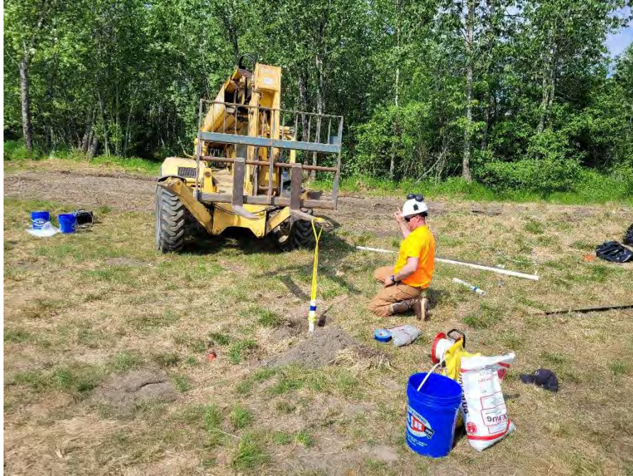
Photograph #1 – 6 June 2022. Paragon staff directs the boom lift operator while decommissioning monitoring well MW1A. One end of the tow strap was hooked to the boom lift fork, and one end was wrapped around the well. A strip of duct tape maximized the bite of the tow strap. View facing northwest.
