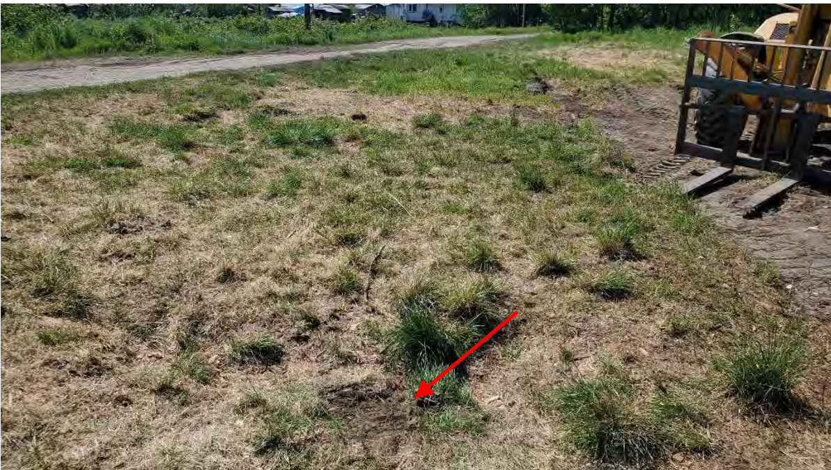
Photograph #4 – 6 June 2022. Decommissioned monitoring well MW2A (marked with a red arrow) after backfilling the soil above the pea gravel. View facing southwest.
