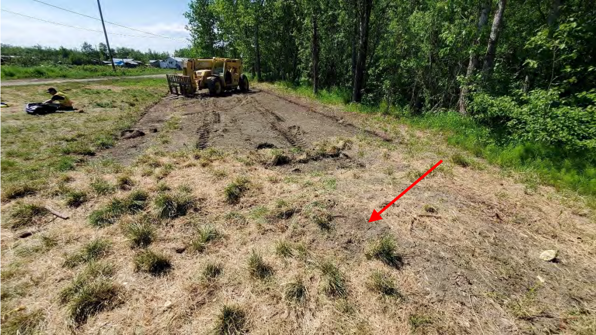
Photograph #5 – 6 June 2022. Decommissioned monitoring well MW3A (marked with a red arrow) after backfilling the soil above the pea gravel. View facing southwest.
