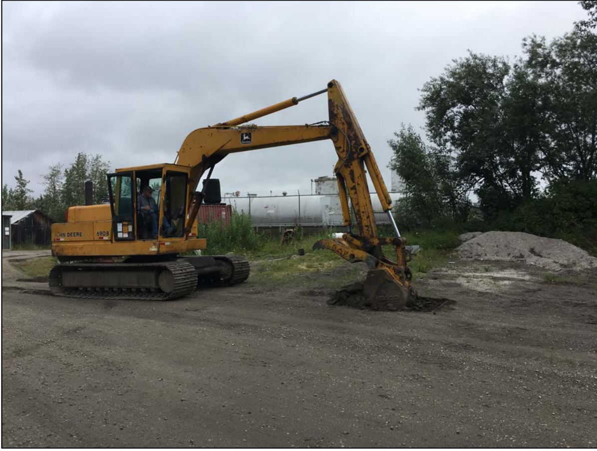
Photo: 1 Date: 8/1/2018 Direction: North Subject: Test Pit #1 and MW-01 location, tank farm in background.
