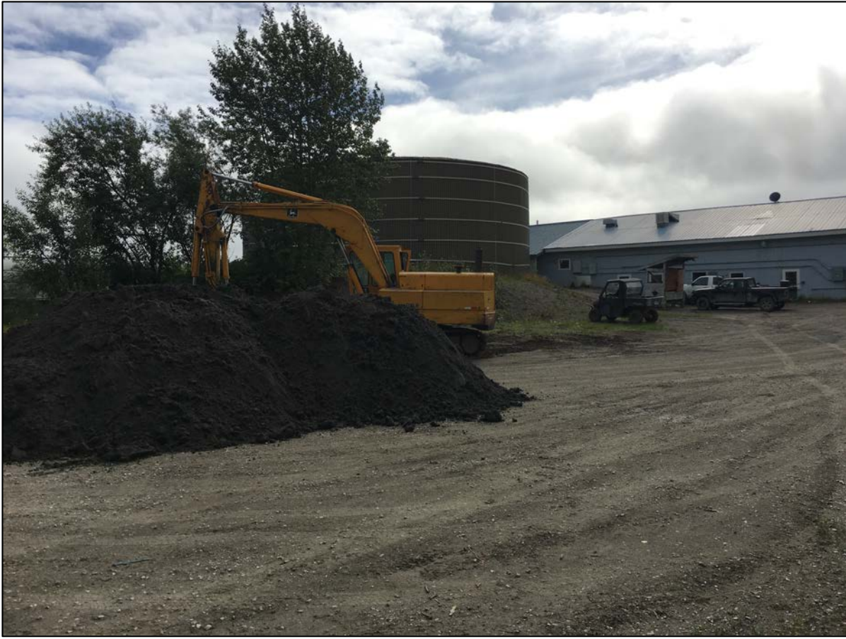
Photo: 3 Date: 8/1/2018 Direction: South Subject: McGrath City Offices in relation to Test Pit #1.
