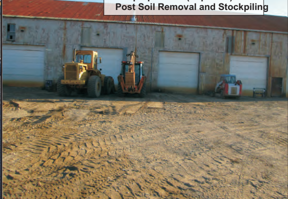
Shop Spill Area (Sep 2014) Post Soil Removal and Stockpiling
