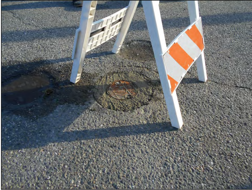
Photograph 15: New Well Cover at MW-29S, Former Park-n-Sell Lot
