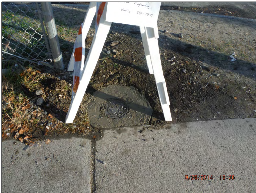
Photograph 18: New Well Cover at MW-27, Southwest Corner of Cushman St. and Airport Way
