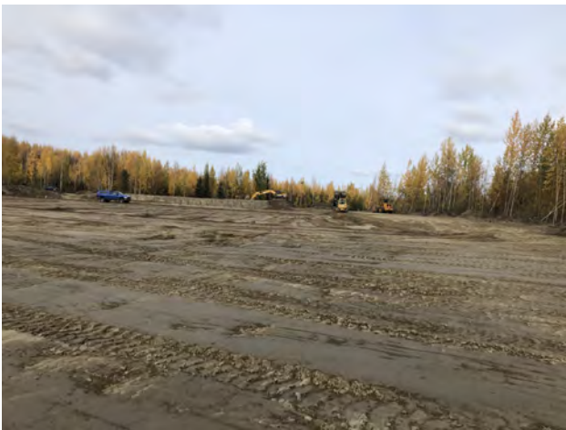
Photo 3: 20210921 Dismantling northern berm
