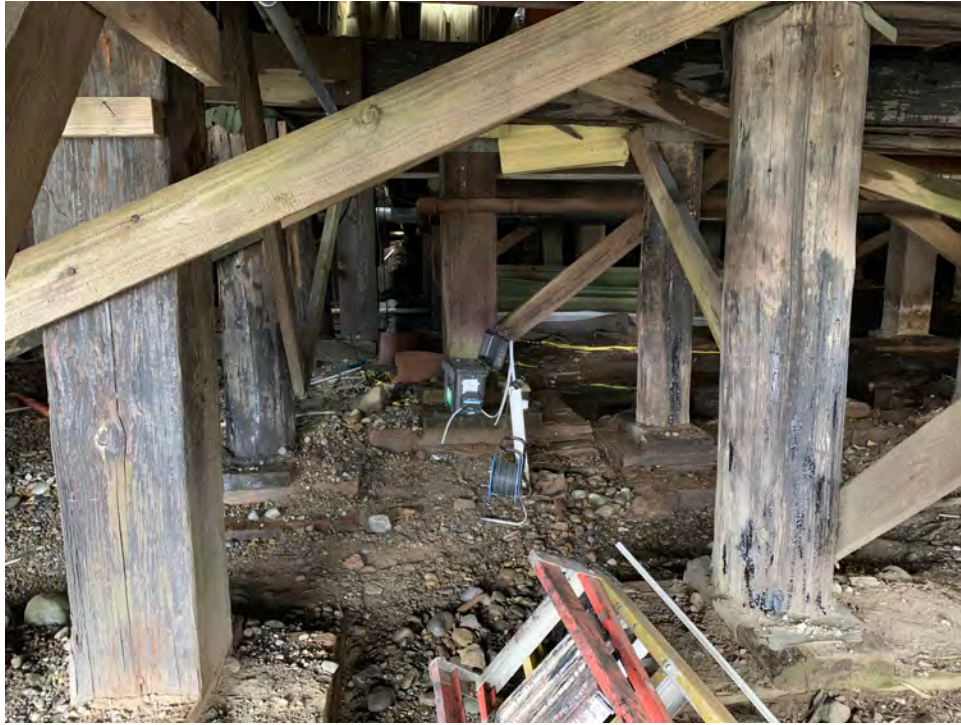
Photo 1: Monitoring Well MW-9. May 1, 2019.
