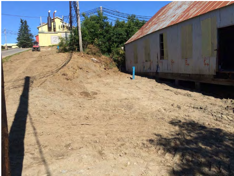
Photo 8: Re-graded excavation area (post-excitation), photo facing north towards completed monitoring wells MW-3 (left, background) and MW-1 (right, foreground)
