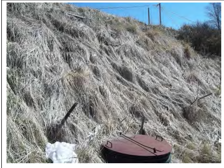
Photo 2: Looking southeast at the stabilized slope above the interceptor trench. Sump 1 in the foreground. (May 12, 2014)
