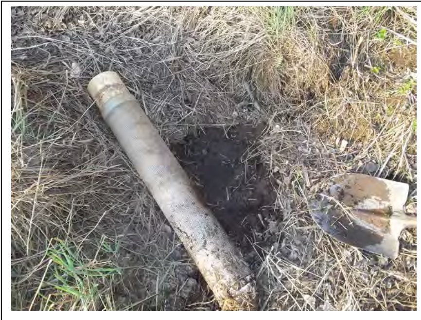
Photo 23: Recovery Well R6 was decommissioned on May 13, 2014 by removing the well from the ground and filling the hole with nearby soil. (May 13, 2014)
