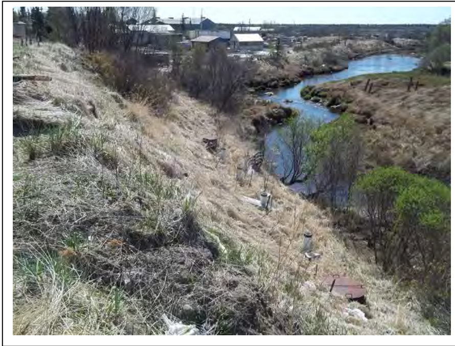
Photo 3: Looking southwest at the re-vegetated and stabilized area in the vicinity of the interceptor trench, with Eskimo Creek in the background. (May 12, 2014)
