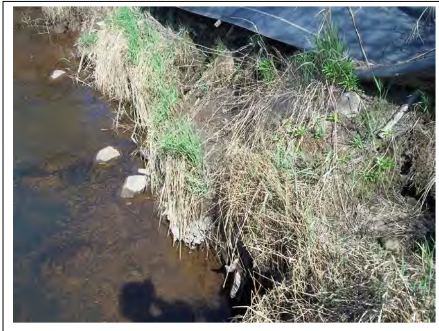
Photo 4: Seeps were not present at the base of the bank where seep samples were previously collected. (May 12, 2014)
