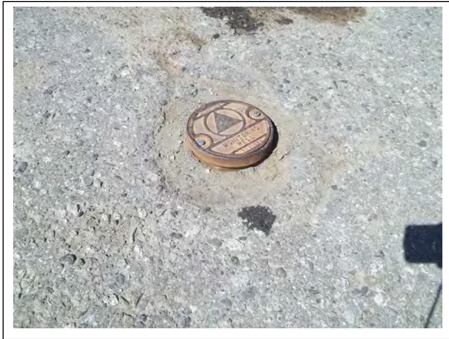
Photo 10: The well casing of Monitoring Well MW-6 was frost-jacked, and the flush-mount monument was loose. (May 12, 2014)
