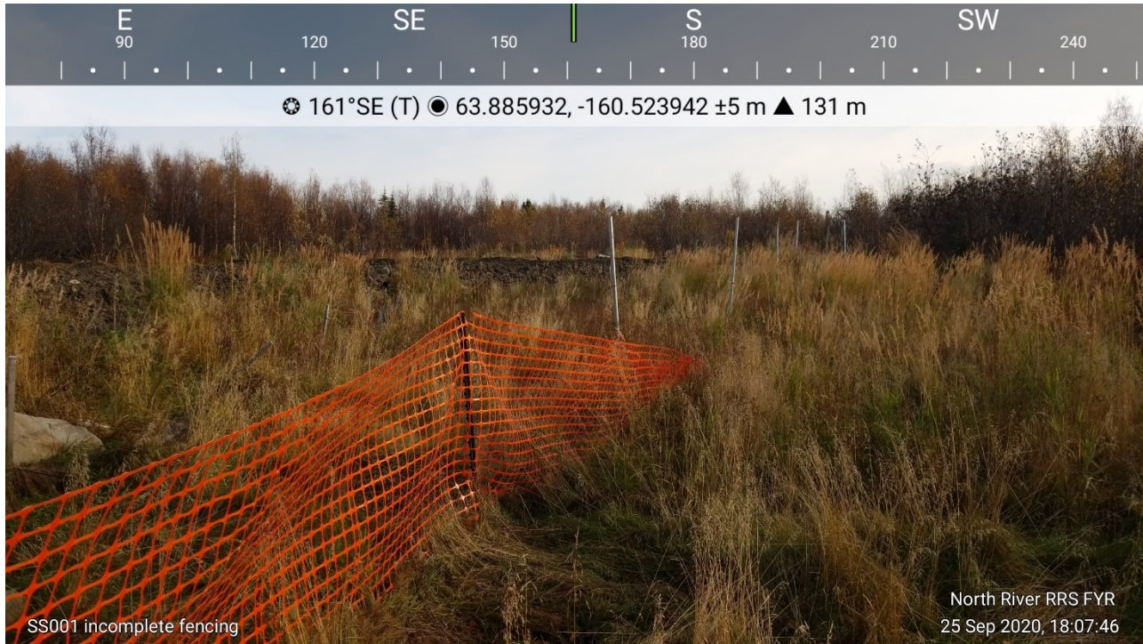
Site SS001 – Incomplete fencing around the site.
