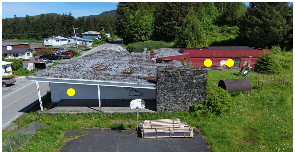
Figure 3 - Photo looking north. White paint and red will be targeted. Door trim may be selected if it is distinctive and readily used elsewhere on the structure. Yellow dots indicate potential paint coatings to be sampled. (Photo courtesy of DEC Solid Waste Program, 2023.)
