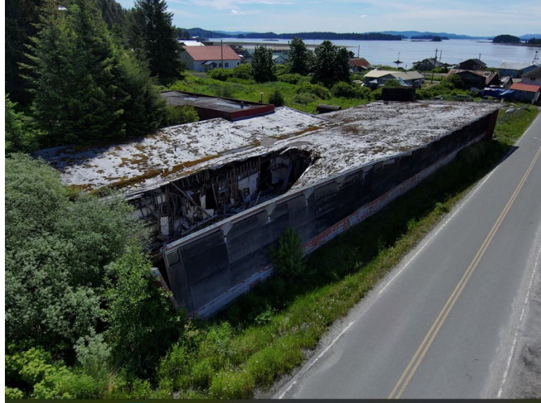
Figure 2 - Looking southeast across top of school, showing collapsed roof in original school structure. (Photo courtesy of DEC Solid Waste Program, 2023.)
