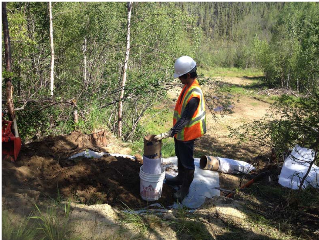
Filling sandbag at IA-2 excavation during removal of west sidewall. View to north.
