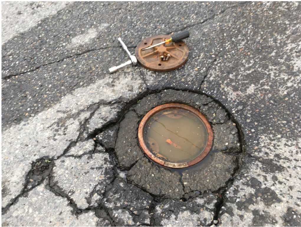
Photo 3: Location of monitoring well MW-34A.
