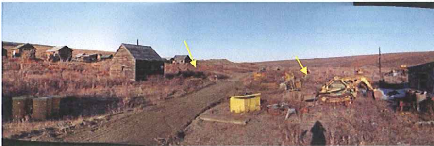
16. Post demolition. Both the carpenter shop and power shed are gone in this photo. Gold house still exists on the left.
