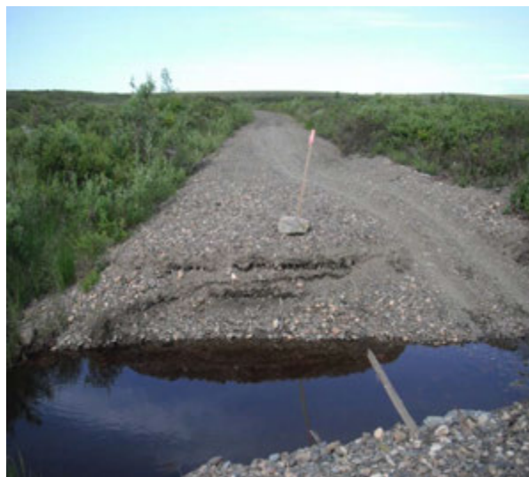
The washout on the Deering to Utica road view looking south on 9/2012
