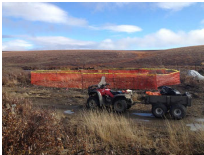
AOC 1 excavation fencing, looking north, as left by the WHPacific Field Crew on 9/23/2012
