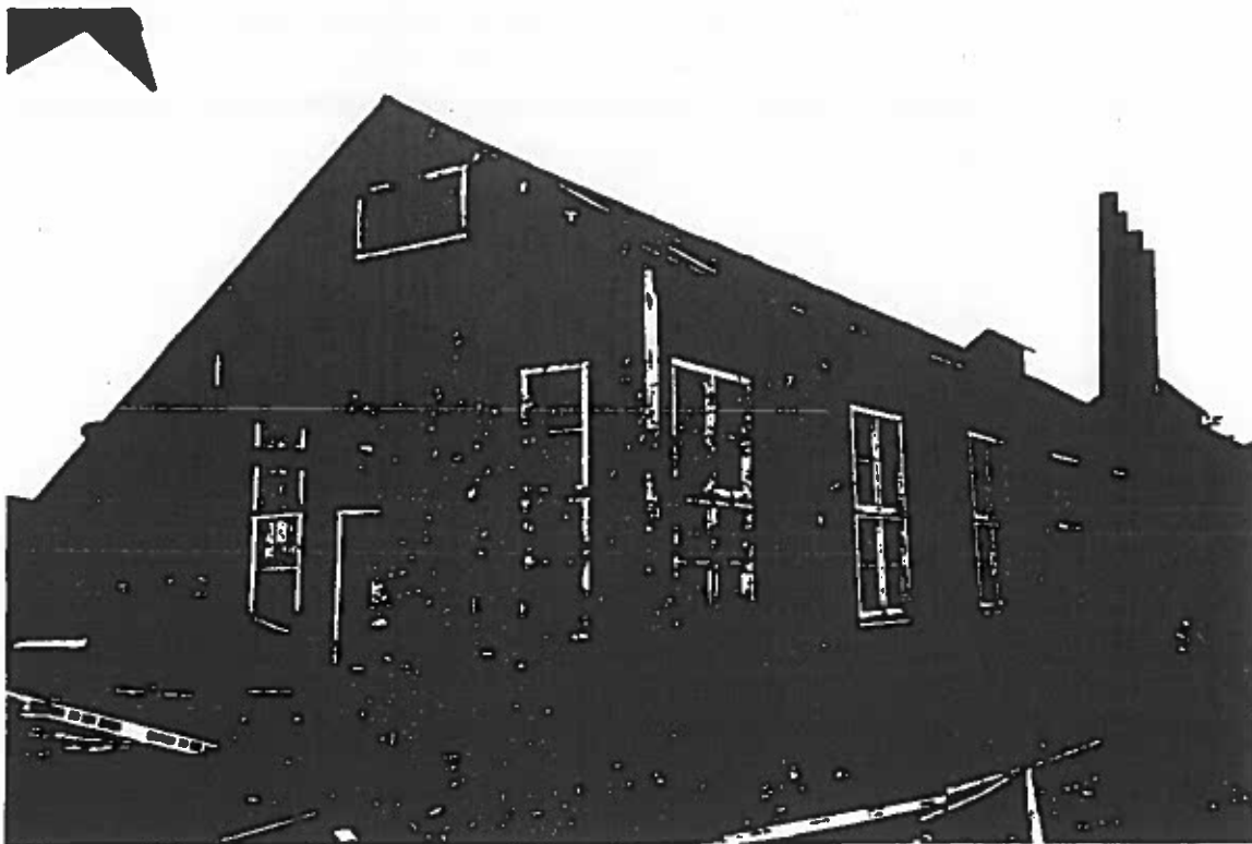
Foundry building with power plant in background. Caution tape is for asbestos removal work.
