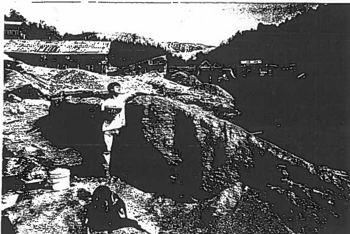
Tailings pile road cut exposing oil layers, looking east. Note darkened oil lenses throughout road cut and stained tailings at left.
