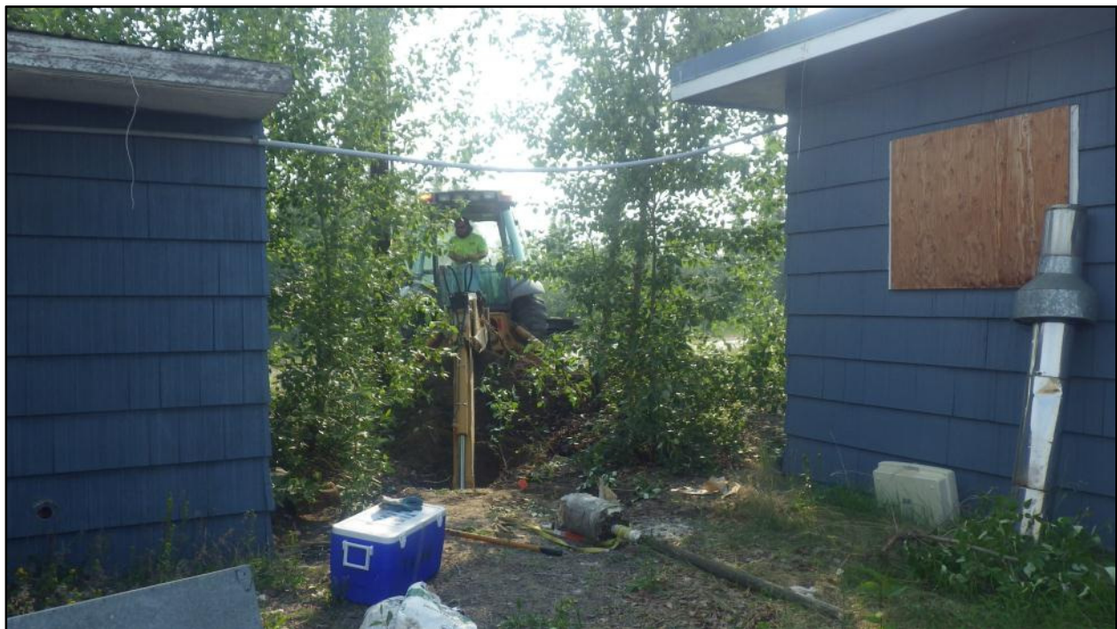
Photograph 6: Excavating test pit 1 at the YFHC. Removed vapor extraction well VE-1 in the foreground(looking west).
