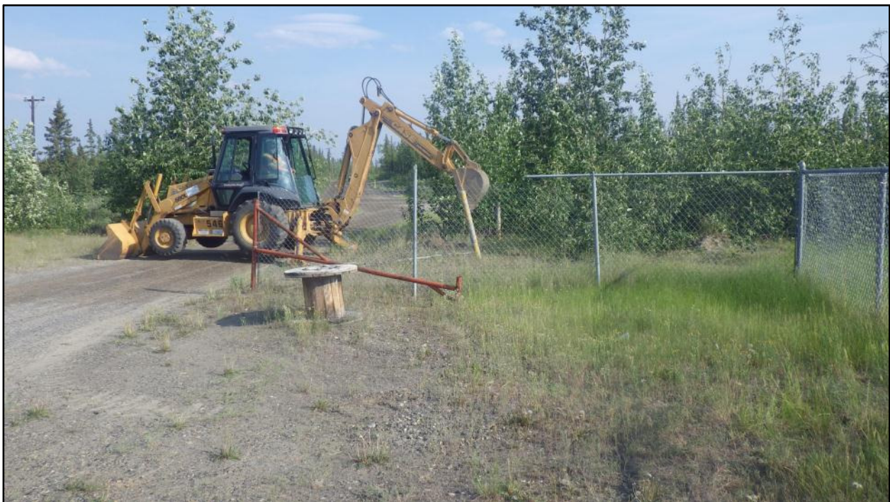
Photograph 4: Backhoe removing protective bollards from former blower house location south of Building 100 (facing south).
