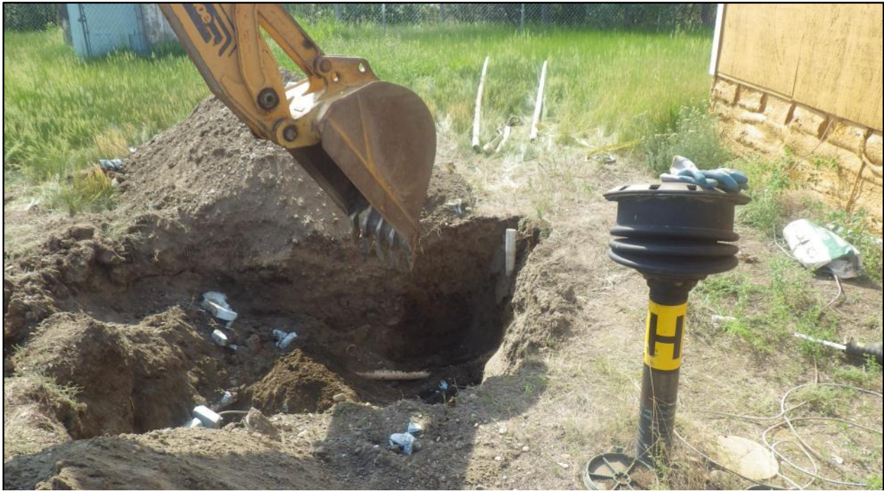
Photograph 3: Exposing air supply pipe in order to cut and cap pipe for removal of sparging well SP-1 (facing west).
