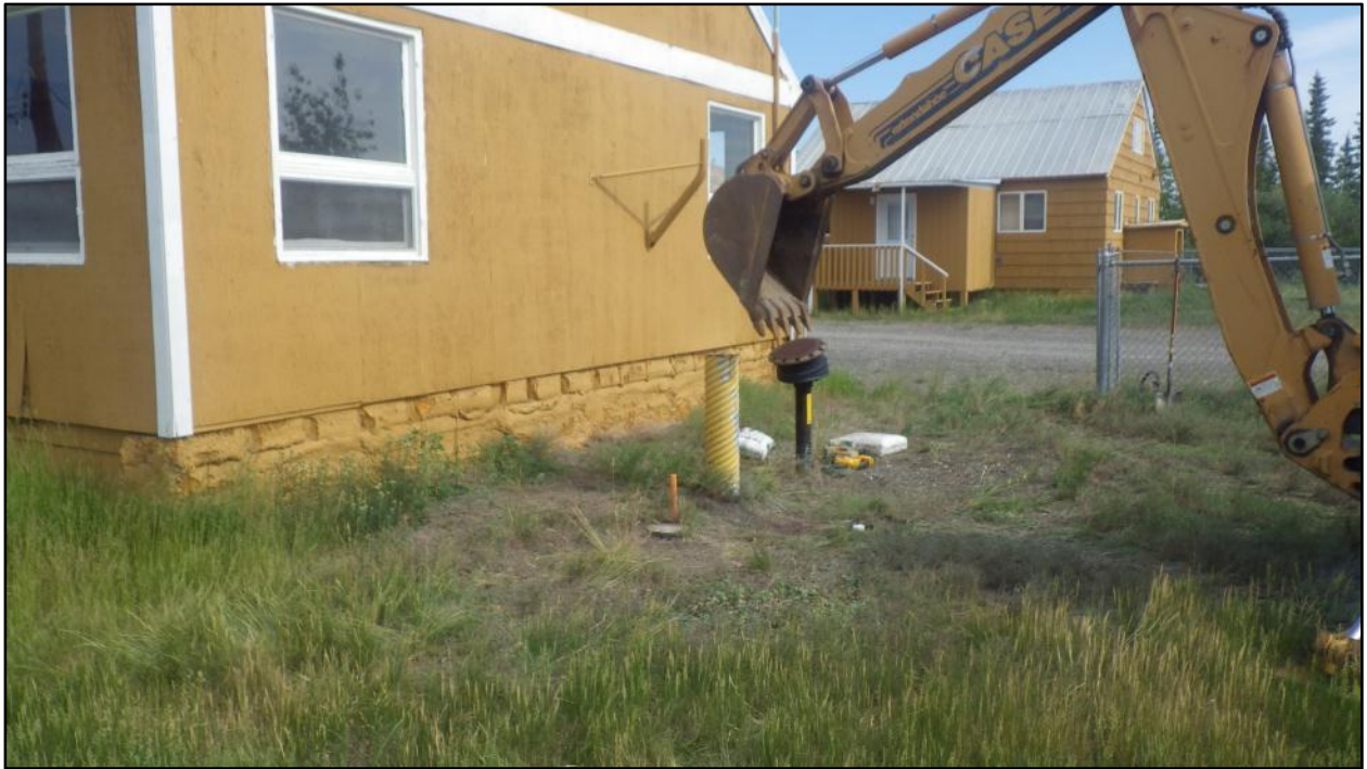
Photograph 1: Building 100 wells prior to decommissioning. UST fill pipe with cover on the right of yellow painted monitoring well protective corrugated pipe (facing northeast).
