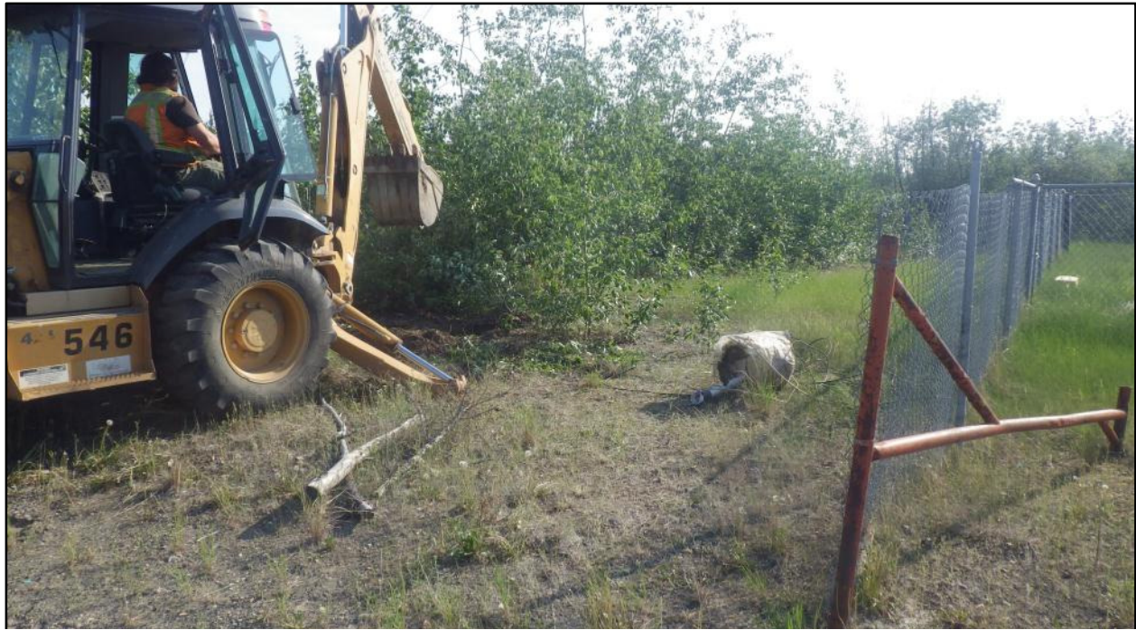
Photograph 5: Removal of remaining air sparging system at former blower house location for Building 100 remedial system(facing southwest).
