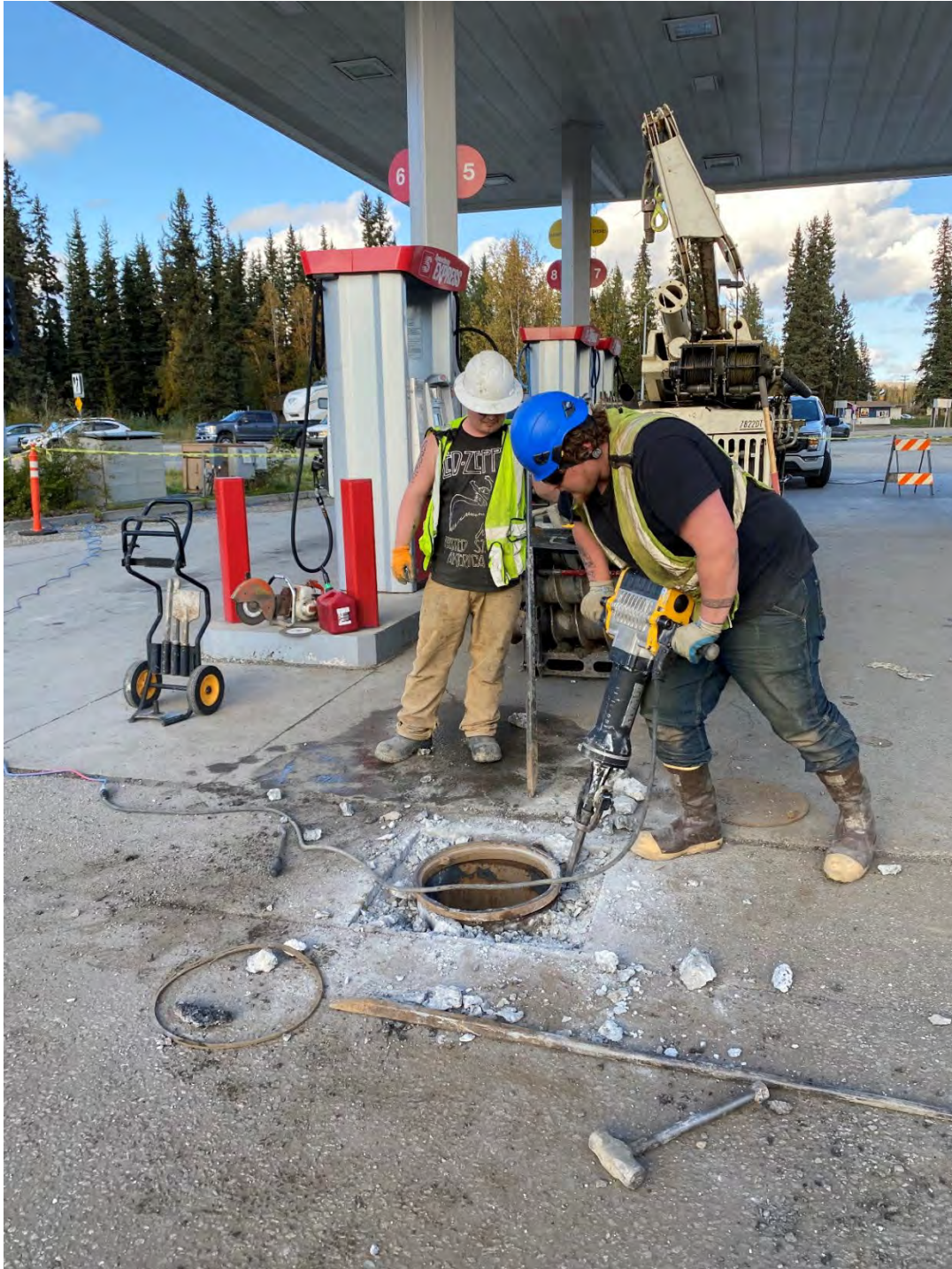
Photo 4: Drillers jackhammering through cement in order to make room for a larger manhole for IW-2023-D.
