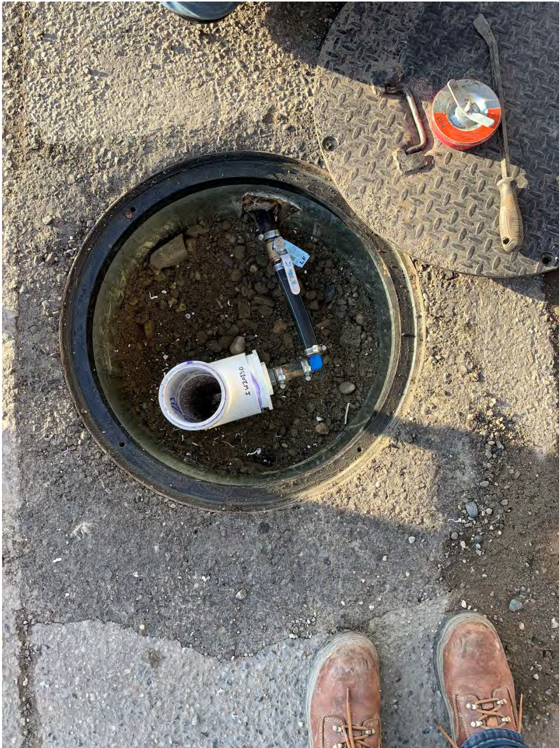
Photo 10: IW-2023-D hooked up to the recirculation system. The area surrounding the manhole was resealed with asphalt after drilling.
