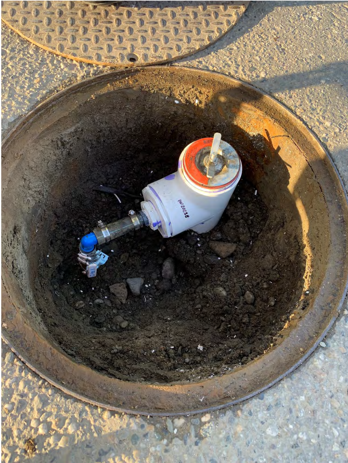
Photo 8: IW-2023-B hooked up to the recirculation system.
