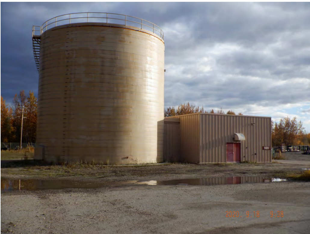
Conducting an IC inspection at OU2; no IC discrepancies were observed in the area surrounding the water supply tank and building (view N)
