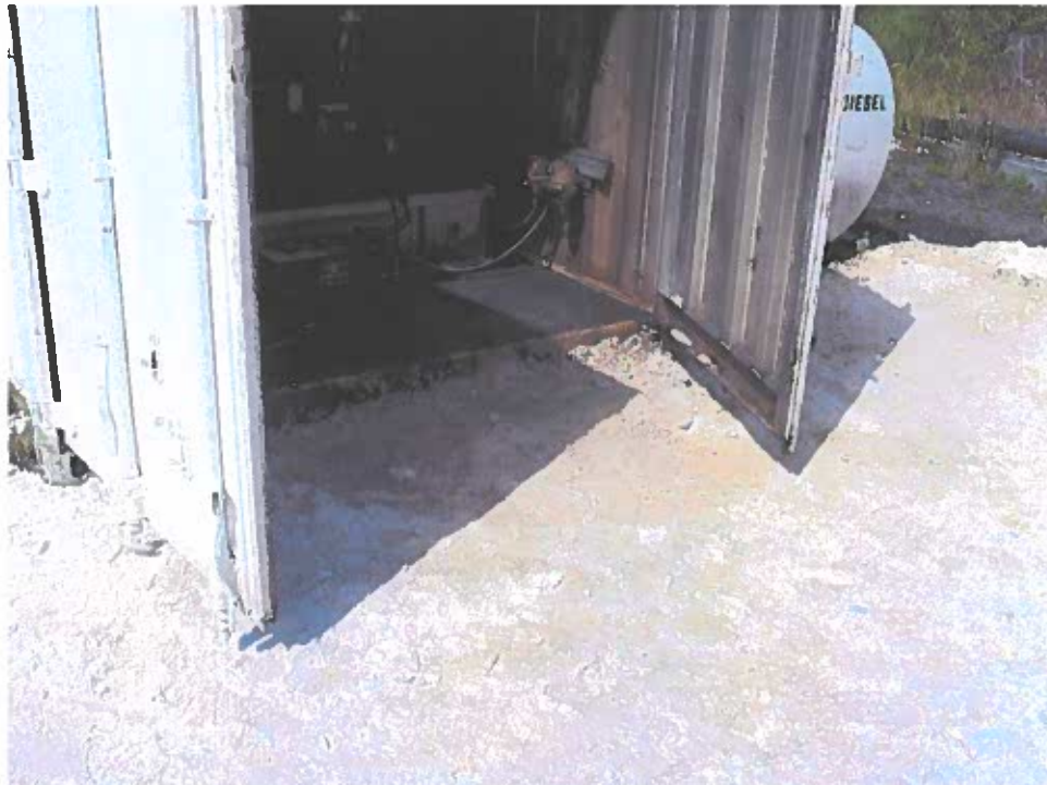
July 31, 2004 Calder Bay Facility, Camp Genset: Close up view of surface staining.
