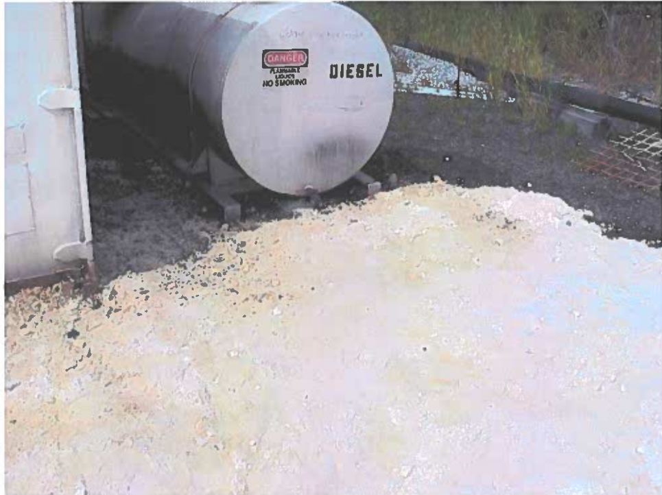
July 31, 2004 Calder Bay Facility, Camp Genset: Close up view of surface staining.
