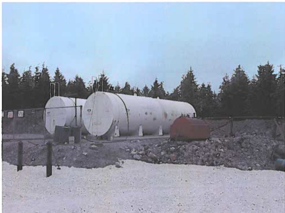
July 31, 2004 Calder Bay Facility, Two 20,000-Gallon Tanks: Surface contamination was observed in front of the right tank extending down the slope to the calcium carbonate in the foreground.
