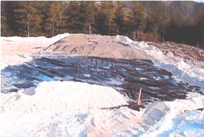
September 2004; Biocell: This view shows biocell construction elements. Cell is about 50% complete.
