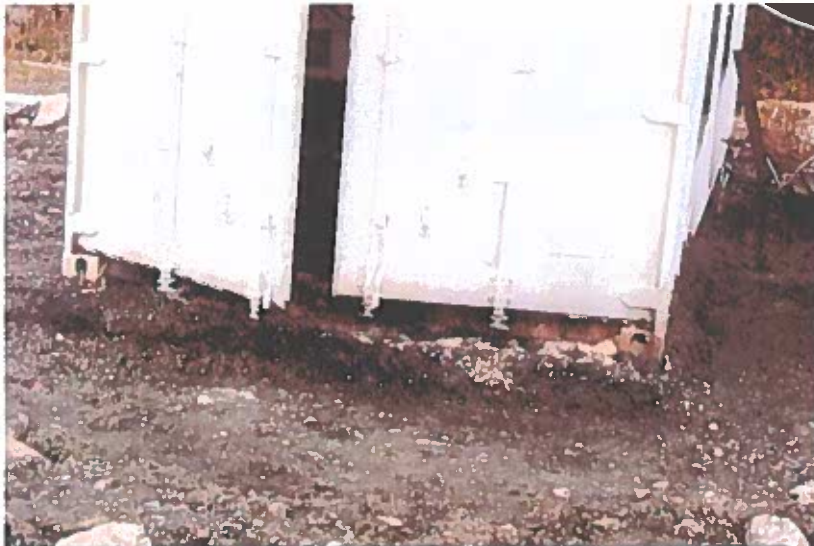
September 2004; Calder Bay Facility, Camp Genset: Close up view showing final depth of excavation of contaminated soil. Contamination left in place beneath genset.
