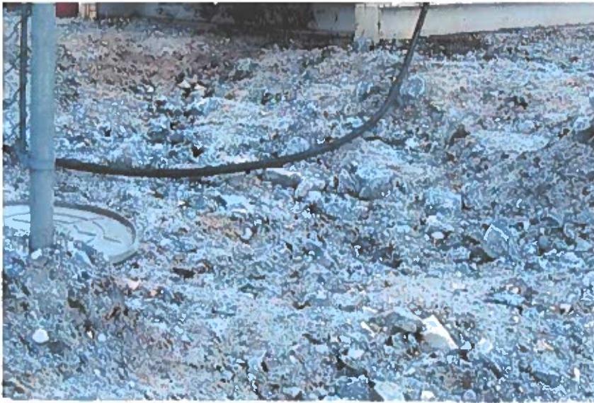
October 8, 2004; Calder Bay Facility, Two 20,000-Gallon Tanks: Close up view showing final depth of excavation of contaminated soil. Note prominence of large shot rock precluding additional excavation.
