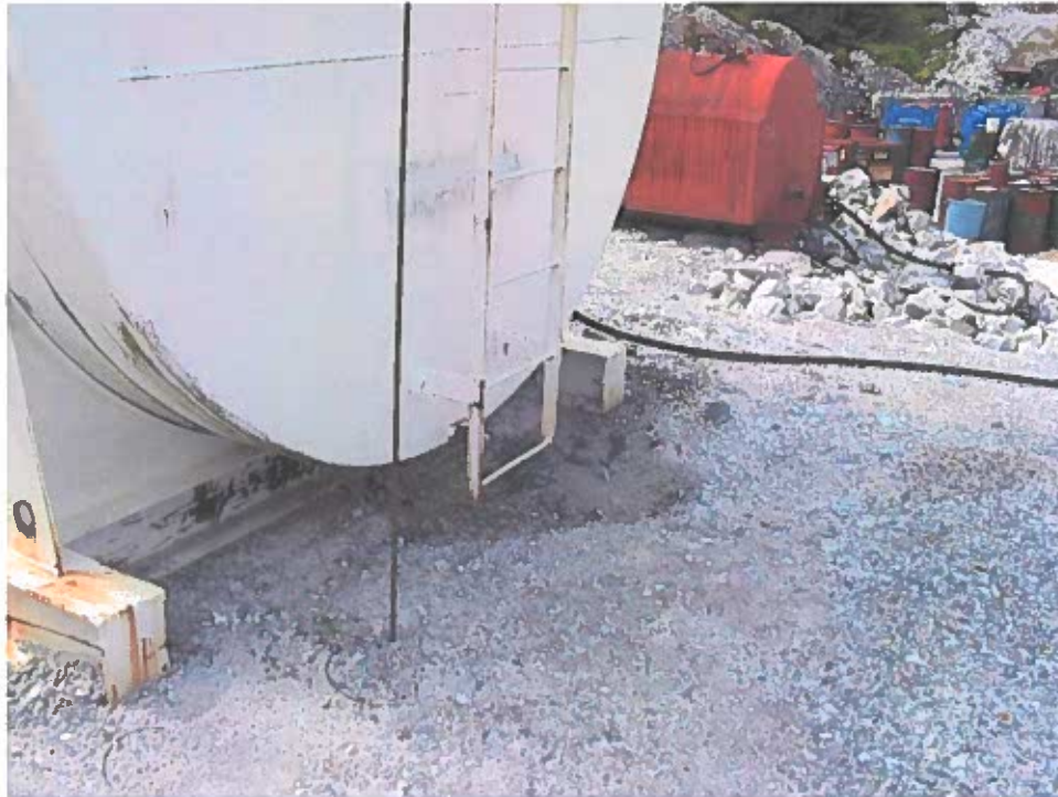
July 31, 2004 Calder Bay Facility, Two 20,000-Gallon Tanks: Close up view of surface contamination.
