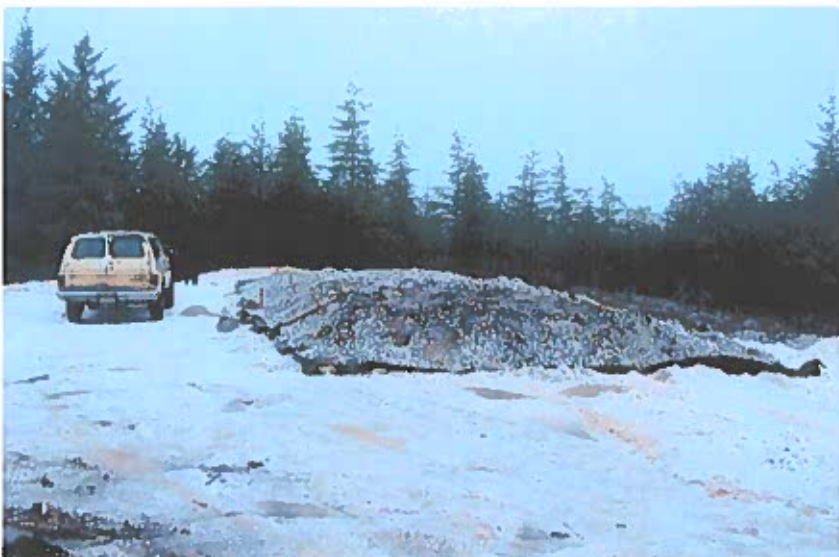
October 9, 2004; Biocell: This view shows completed biocell after about one month of operation. No seepage of oil was noted from cell.
