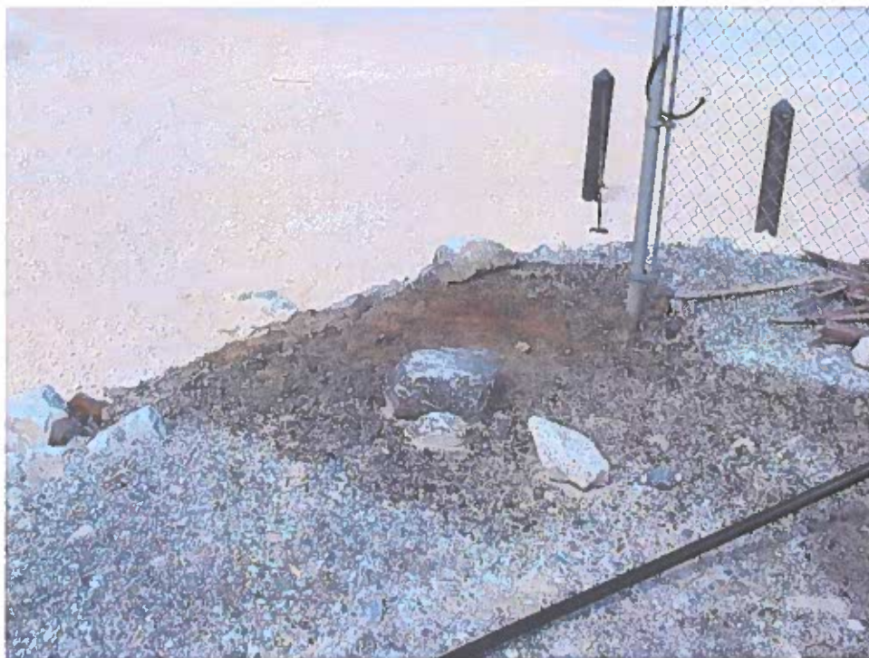
July 31, 2004 Calder Bay Facility, Two 20,000-Gallon Tanks: Close up view of surface contamination extending down the slope to the calcium carbonate.
