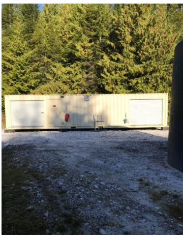
Photo #17 Area in between Camp Generator & Poly Tank
