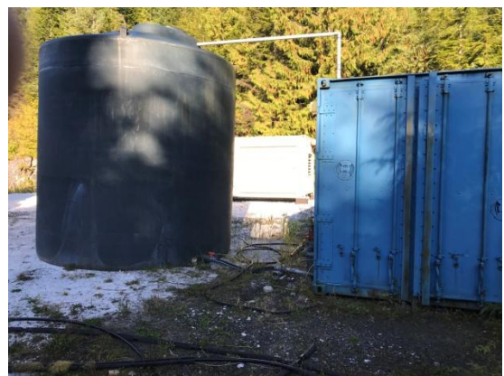
Photo #18 Water Treatment Unit & Poly Tank with Camp Generator in background
