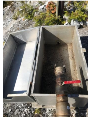
Photo #2 Header Spill Containment
