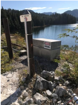
Photo #1 Fuel Header
