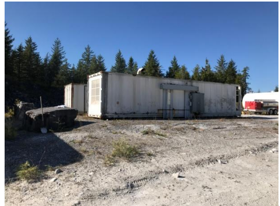
Photo #4 Twin Diesel Generators Fueling Station
