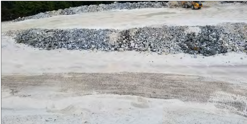
PHOTO 21 HydroCon2 Stockpile Thinly spread treated soil from HydroCon2 stockpile at the Rock Dump.
