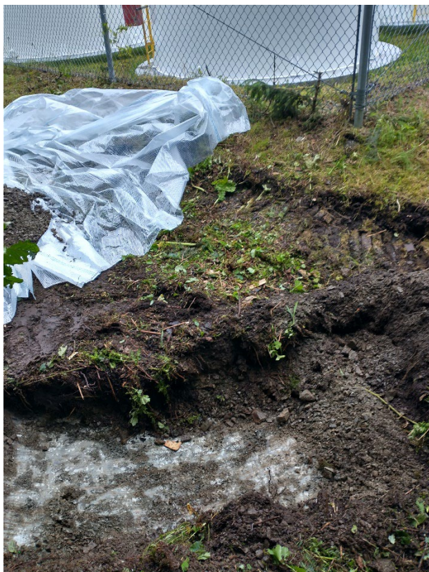
Photo 4: Test Pit TP3, view Diesel ASTs, view northwest. (July 19, 2023)
