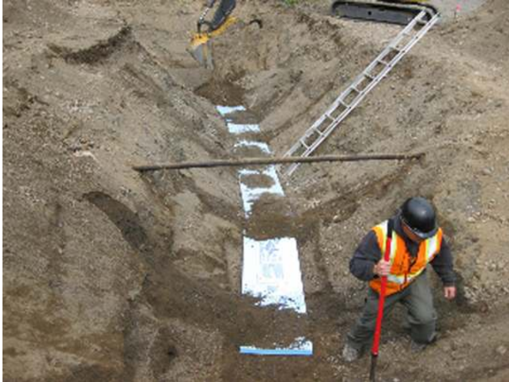
A worker lays blueboard insulation above a newly installed water distribution main for Nikishka Bay Utilities in Kenai. The $2.1 million project was part around $40 million in stimulus funds distributed through the Alaska Department of Environmental Conservation. (More photos available, upon request.)
