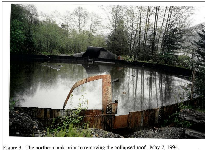
Figure 3. The northern tank prior to removing the collapsed roof. May 7, 1994.
