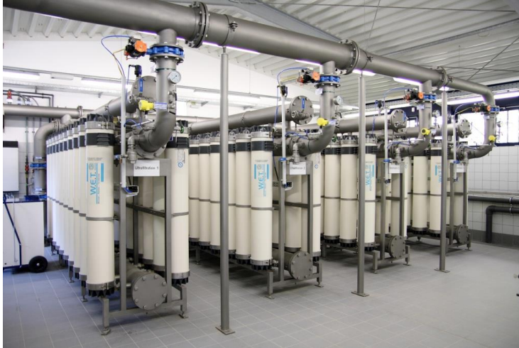
Figure 32 (Courtesy of Enviro Tech)
