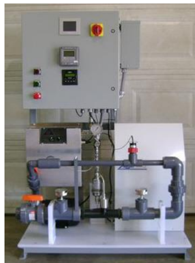
Figure 52 (Courtesy of Absolute Ozone - Water Treatment System)
