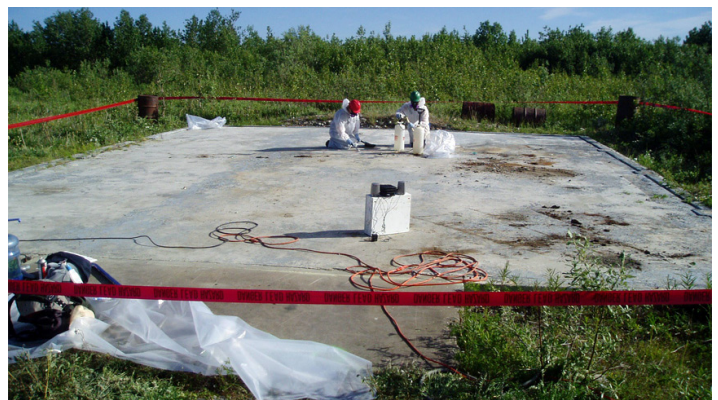
Lead paint is removed from concrete prior to demolition at a site in King Salmon, Alaska
