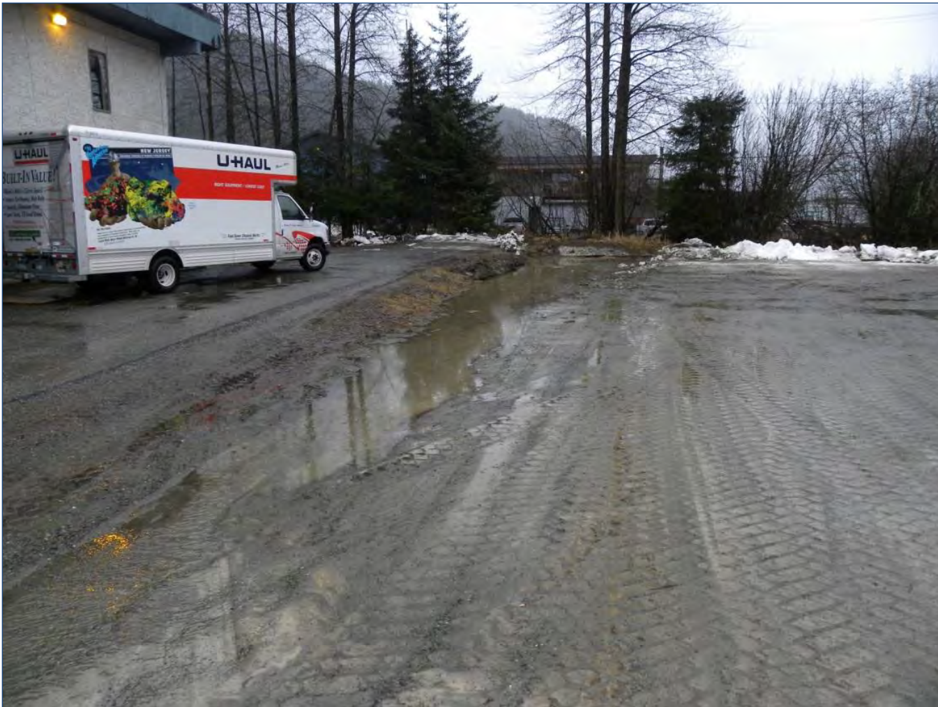
Figure 6. The Edward K Thomas Building project site during a rain event with stormwater run-off draining towards Jordan Creek, which is in the background.
