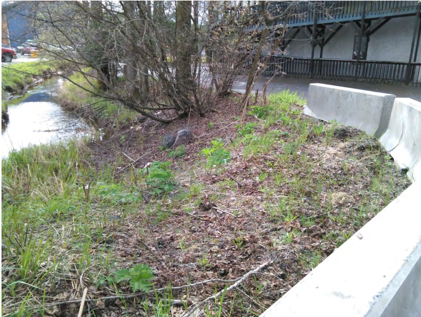
Figure 32. Spring assessment of riparian plantings at the front corner of the property. Winter plowing caused the leaf and sediment deposits prior to placement of the concrete barriers. However, this location was not as impacted as the back corner from last winter. Photos taken by JWP on April 15, 2016.
