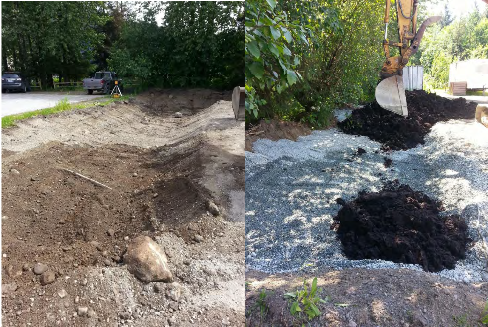
Figure 35. Construction of the rain garden and rock swale continues. The rock swale excavation (left) and placement of drain rock and top soil in the rain garden (right). Photos taken by Dave Hanna, SOURCE, LLC., on June 9, 2016.
