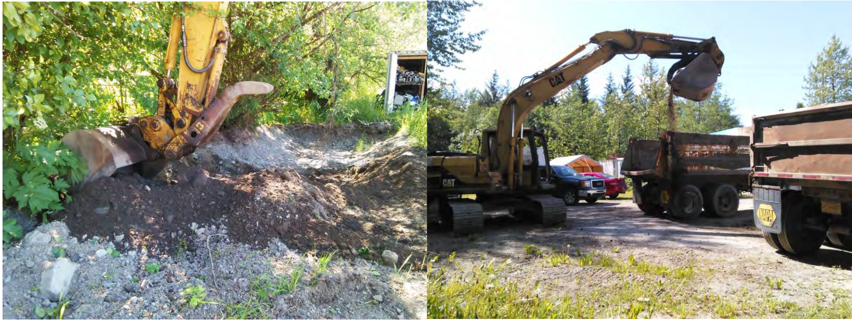
Figure 34. Start of the final construction of the rain garden on May 28, 2016. Photos taken by JWP.
