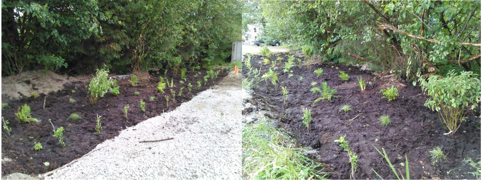
Figure 38. Photos of the completed rain garden from different angles. Photos taken by JWP on June 11, 2016.
