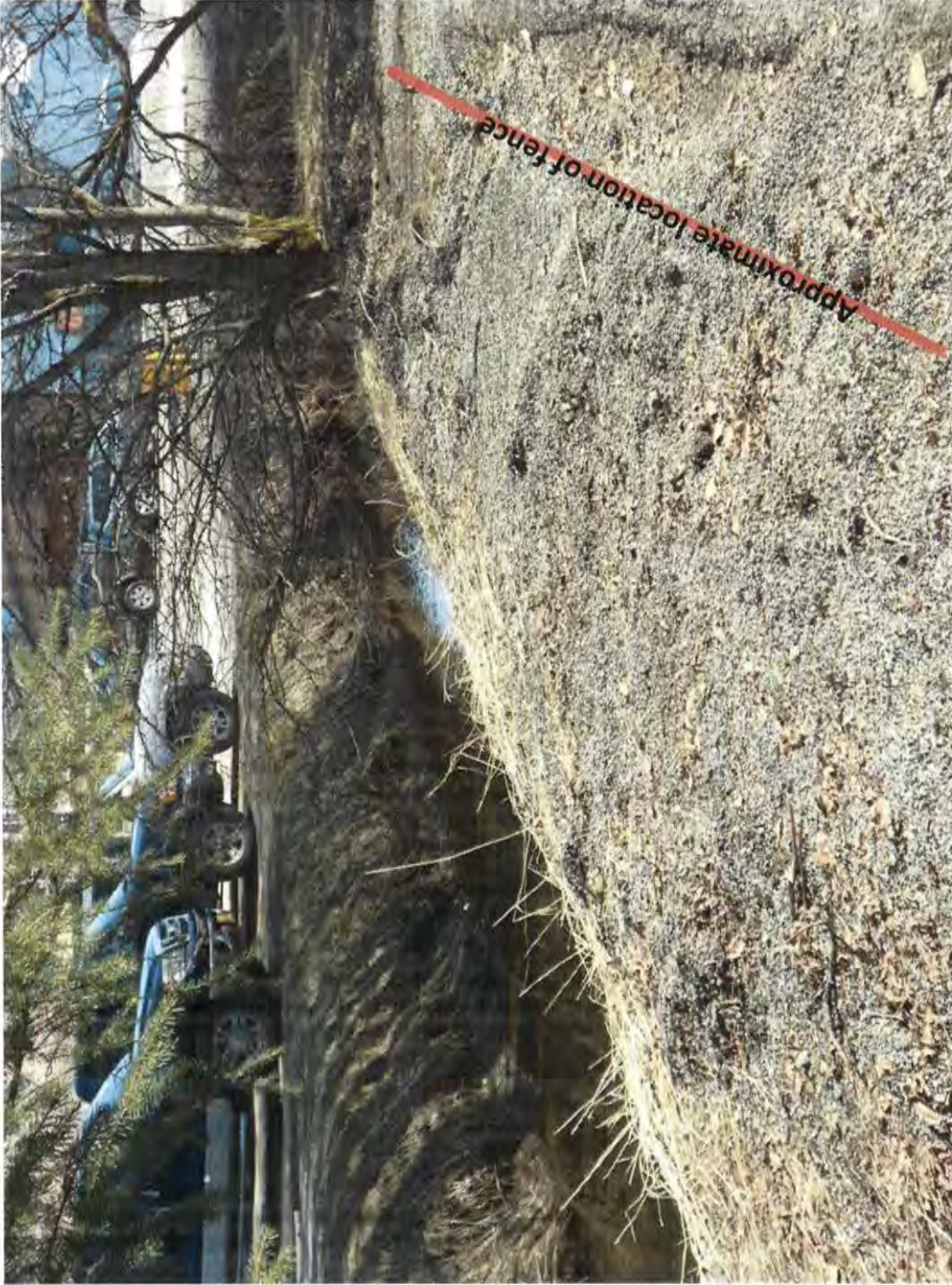
Figure 7. North side of the Edward K Thomas Building, looking east toward back parking lot. Concrete barrier will be placed along the edge of pavement within the vegetation (not yet emerged in this photo) due to risk of impact from plow; however, this length may be replaced with split rail fence depending on funds and land-owner preference.
