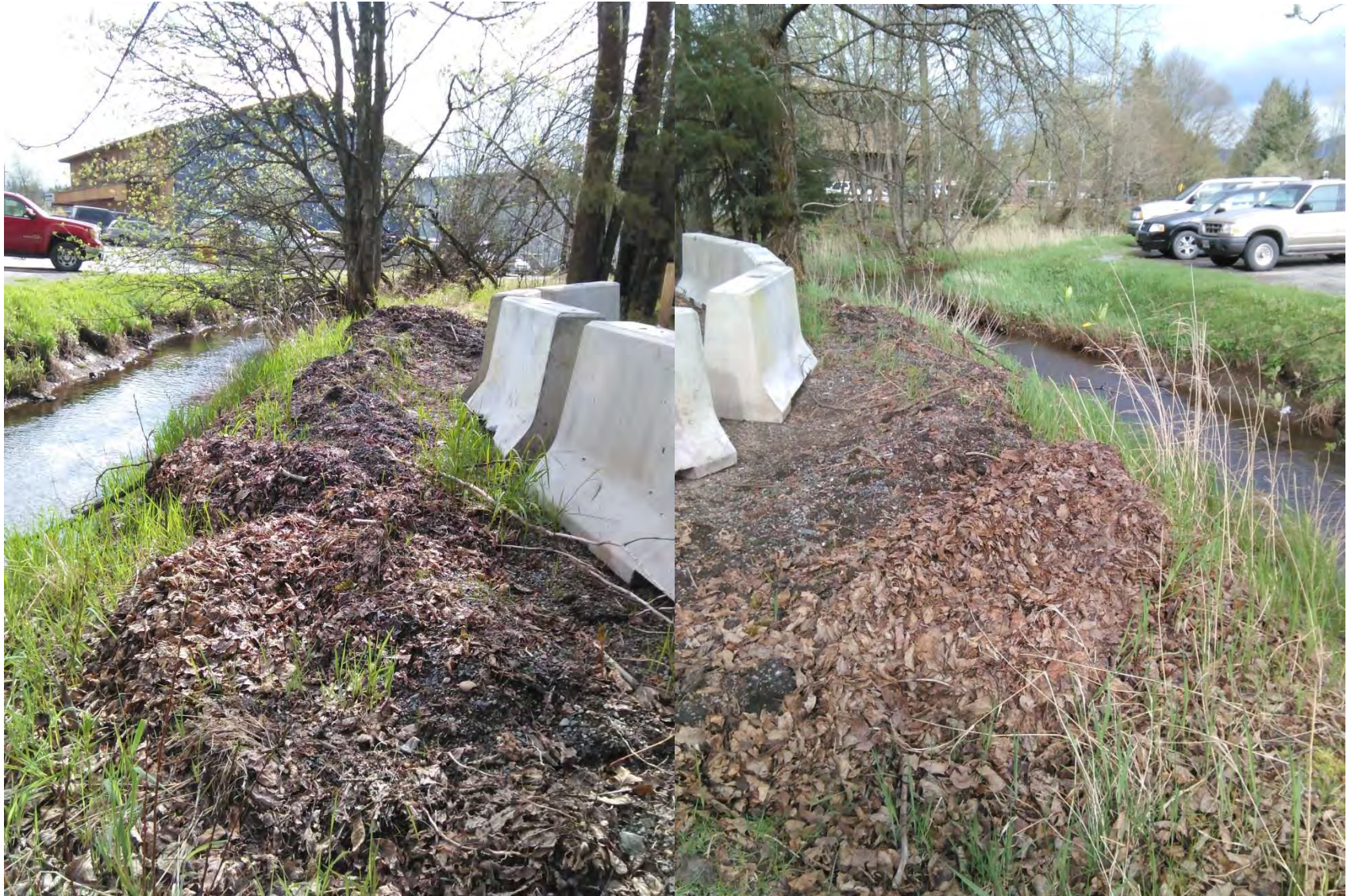
Figure 30. Spring assessment of riparian plantings at the back corner of property looking downstream (left) and upstream (right). Winter plowing caused the leaf and sediment deposits prior to placement of the concrete barriers. This location is the most impacted from last winter. Photos taken by JWP on April 15, 2015.
