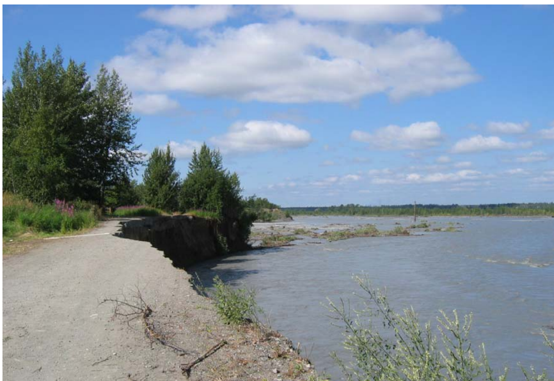
The bank erosion has started to impact the local roadway. Notice the trees that have fallen into the Matanuska River just downstream of the cut bank. (7/16/04)
