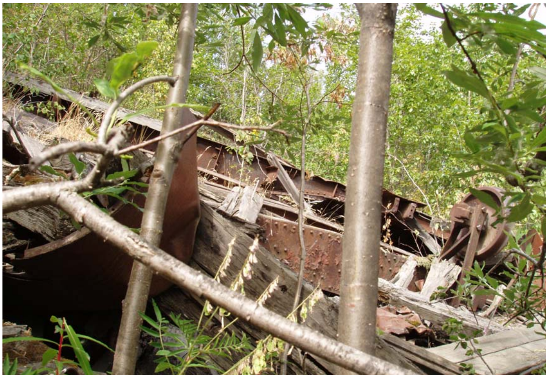
Photo showing rail car debris intermingled with trees and other vegetative growth. (7/16/04)
