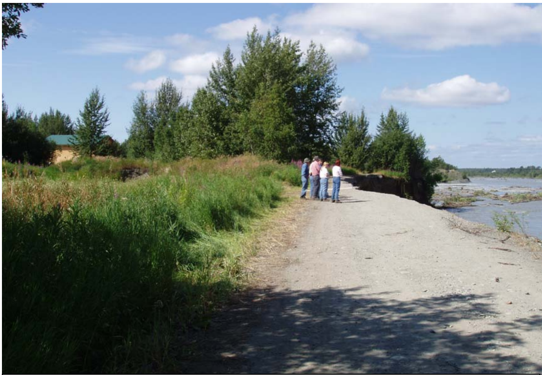
Active Matanuska River bank erosion is occurring in the Circle View Estates subdivision just downstream from protective dikes. (7/16/04)
