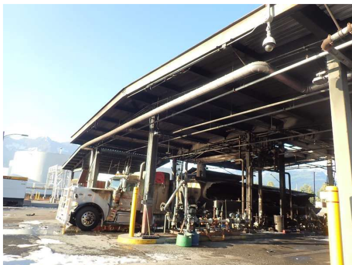
Photo by ADEC 06.27.22 Tanker truck after the fire extinguished at the Truck Loading rack
